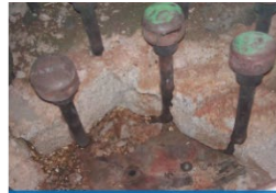
Fluid Bed Incinerator Air Distribution
