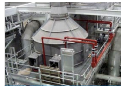
Wet ESP Improvements
