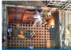
Baghouse Stainless Steel Liner
