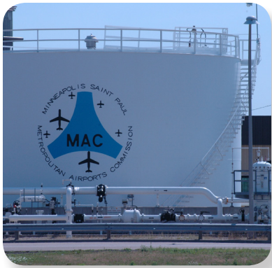
Figure 10-6: Fuel farm at MSP
