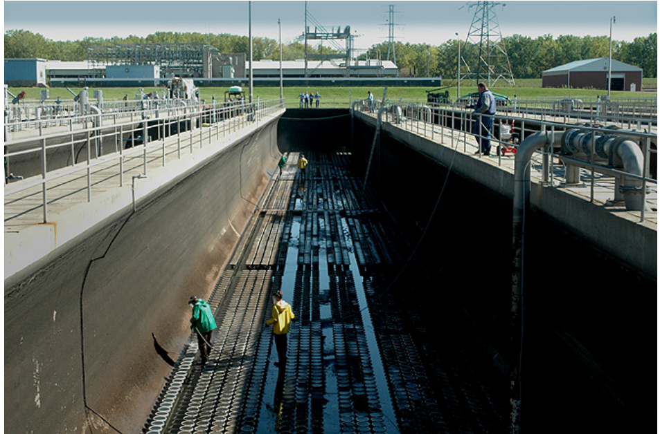
Workers used high-pressure water hoses to clean off the fine-bubble air diffusers at the bottom of a large treatment tank at the Metro Plant.
