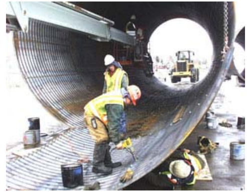
Workers assemble a 16-foot-diameter steel cylinder that will form the wall of a vertical shaft extending 76 feet underground. At the bottom of the shaft, another crew will bore a tunnel through the ground and install the new sewer pipe.
