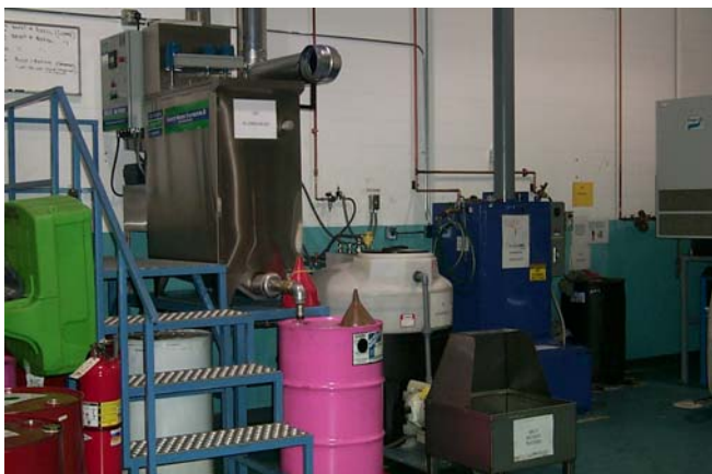
Evaporator installed at Parker-Hannifin Chanhassen facility
