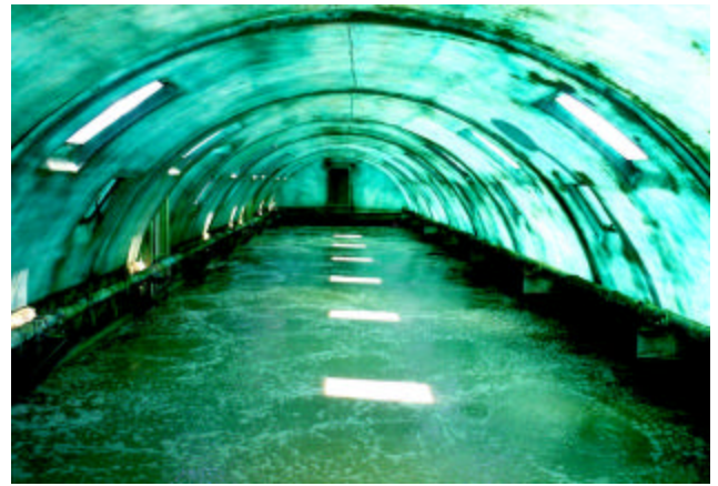
Inside view of the Bio-P anaerobic tank
