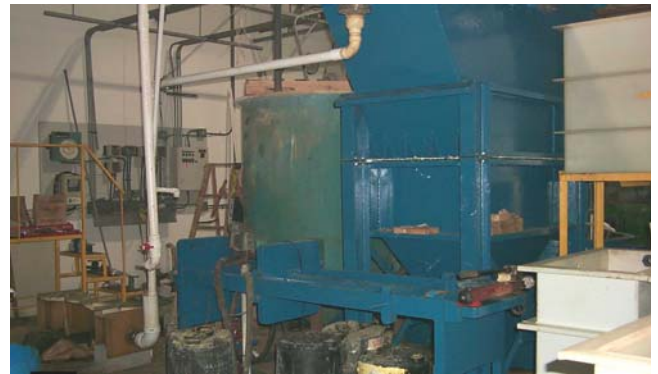
Pictured above is the dysfunctional pretreatment system installed at Prime Plating Inc. The company chose to bypass this system and violate their wastewater discharge permit instead of stopping production long enough to repair or replace the system.
