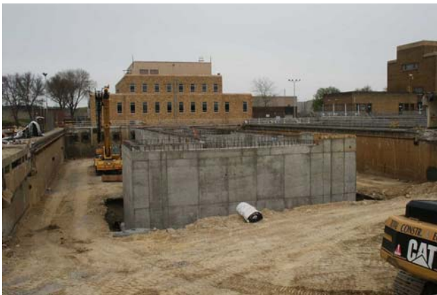
Construction of the new liquid waste disposal site at the Metropolitan Wastewater Treatment Plant.
