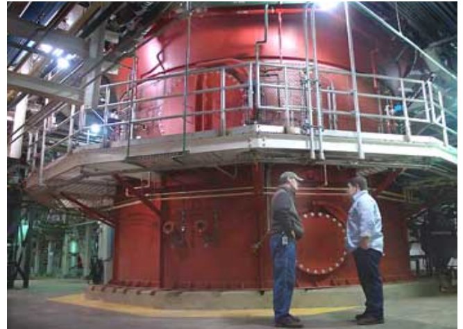
Two Metro Plant employees conferring at the base of one of the three fluidized-bed incinerators.
