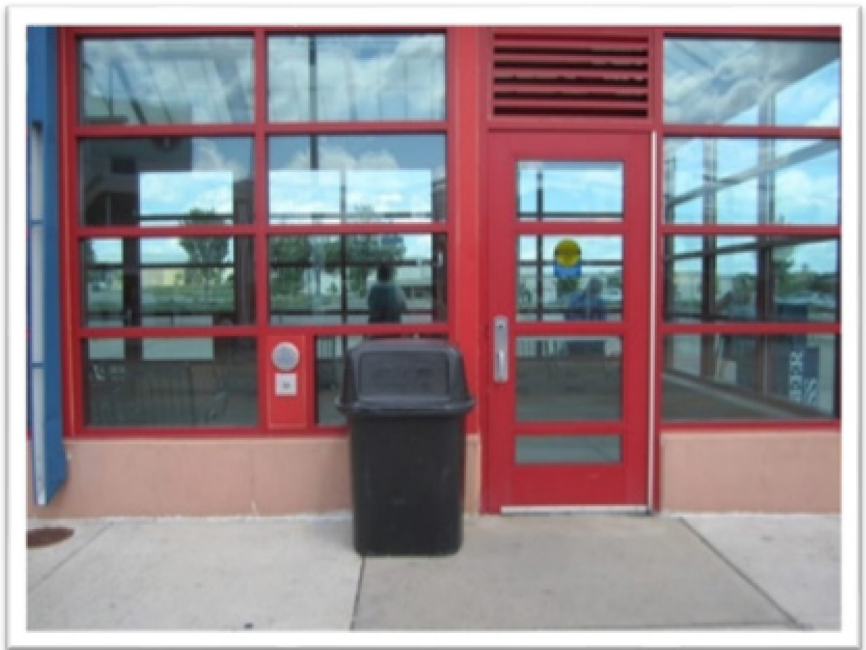
The top photo is an example of a simple fix that requires Metro Transit public facilities staff to relocate the receptacle to make the power-assisted door functional.
