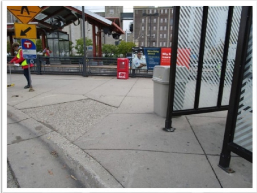
The top photo shows a cross slope of 8.1% (above the 1:48 threshold required by American National Standards Institute 403.3). This is an example of a complicated fix since the bus shelter is connected to heat and light and cannot be easily relocated.
