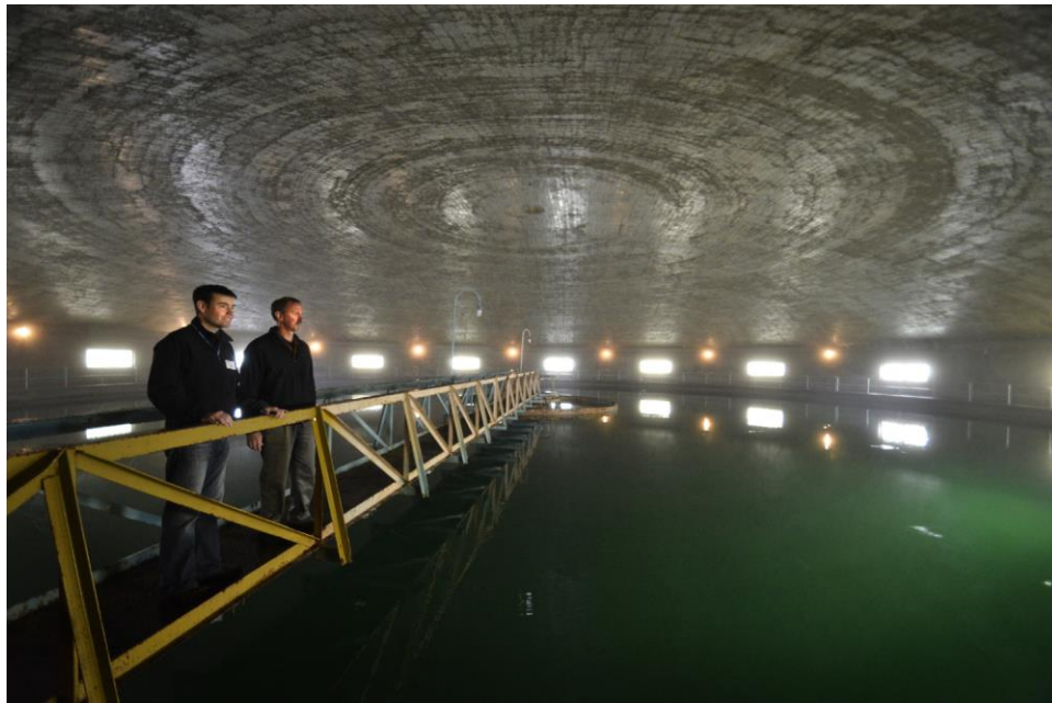
Inside the Clarifier at St. Paul Regional Water Services Treatment Plant. Source: Metropolitan Council Digital Image Library
