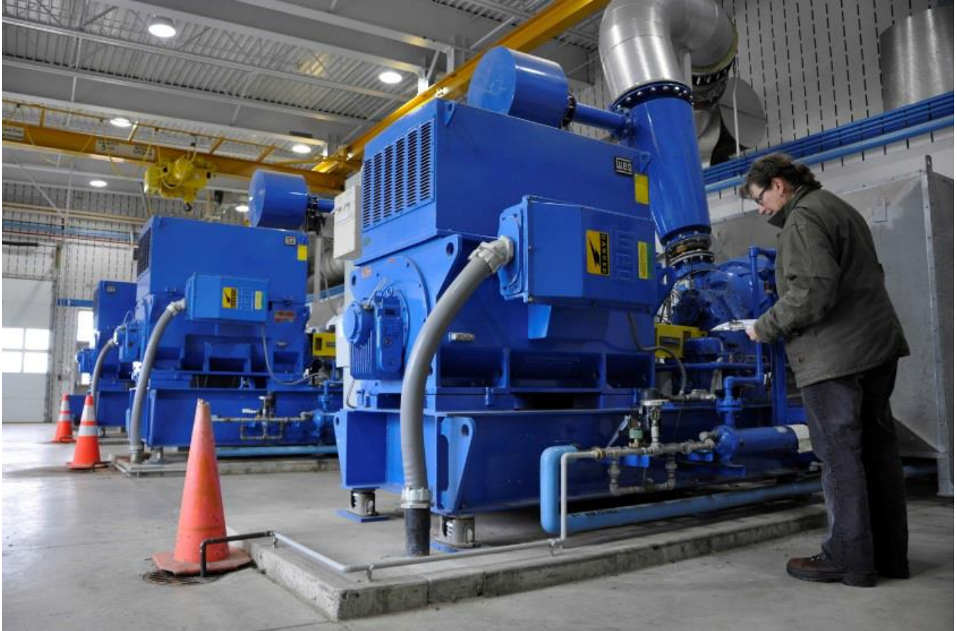
Auxiliary equipment provides backup service at MCEs WWTPs during floods, power outages and other emergencies. Source: Metropolitan Council Digital Image Library
