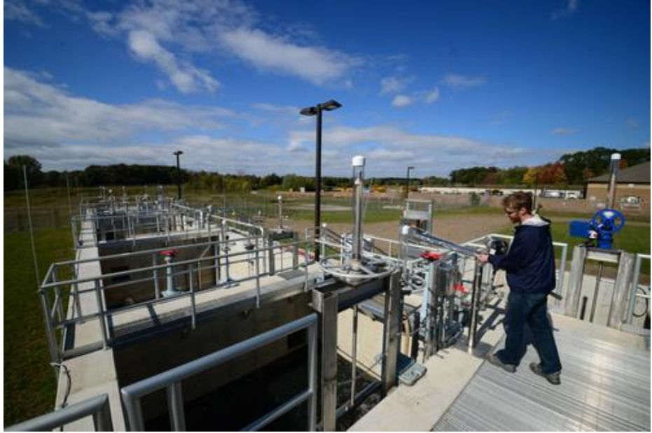
East Bethel WWTP & Water Reclamation Facility. Source: Metropolitan Council Digital Image Library
