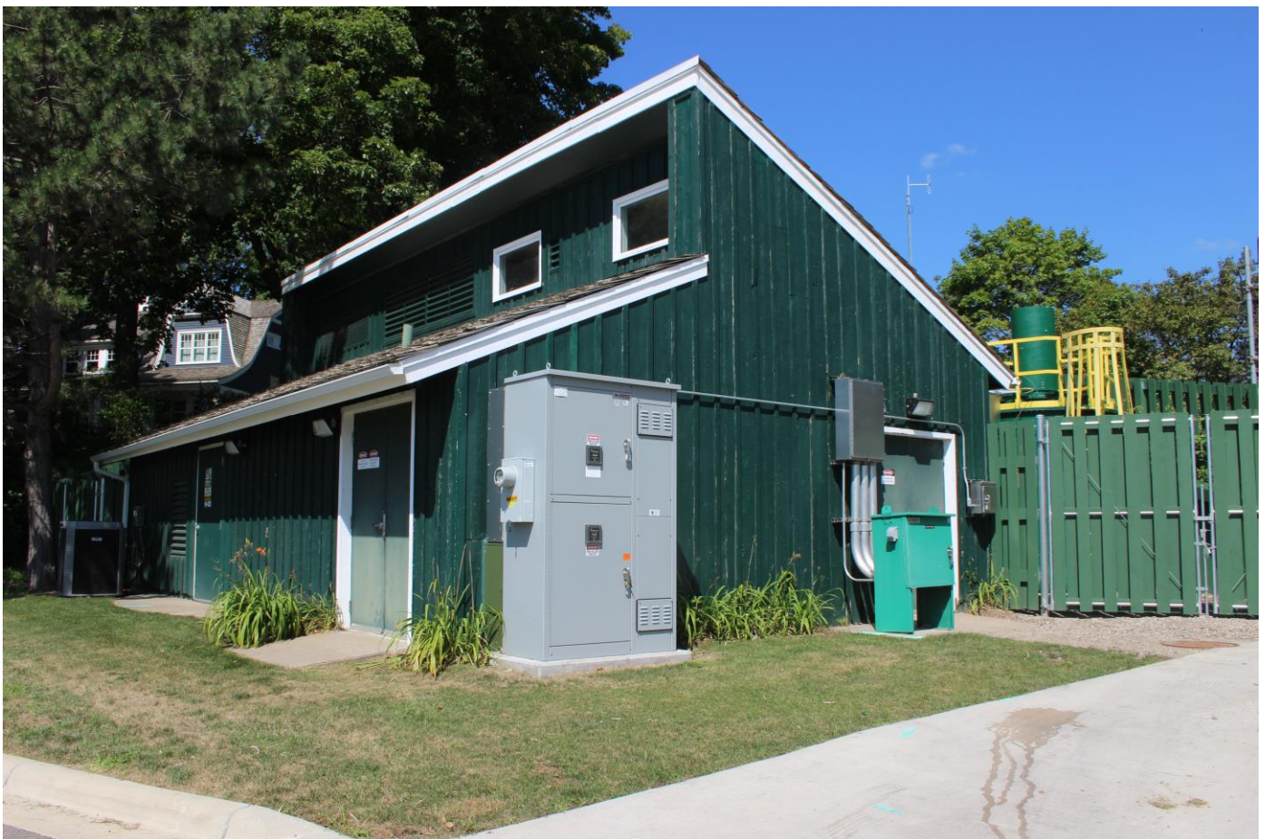
Lift Station. Source: Metropolitan Council Digital Image Library
