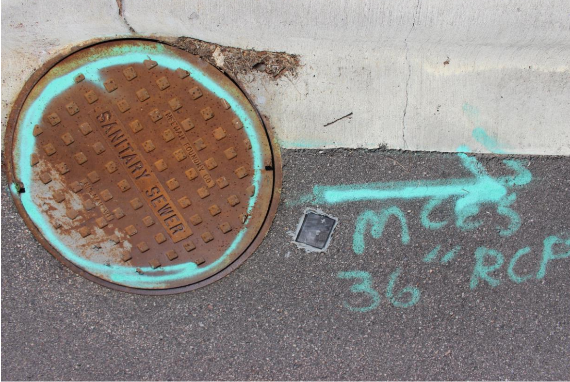
Sanitary sewer maintenance hole. Source: Metropolitan Council Digital Image Library
