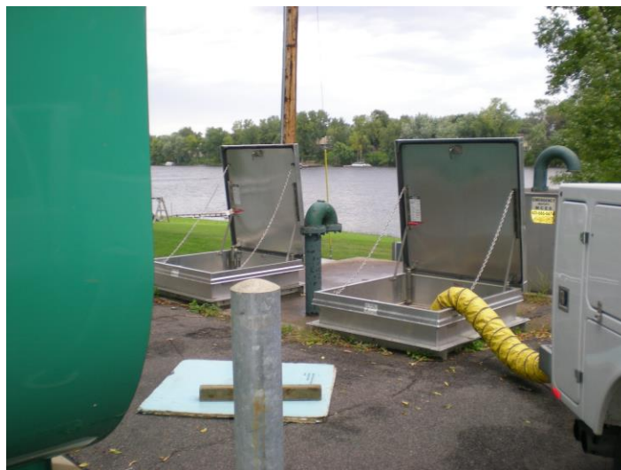
Meter Vaults. Source: Metropolitan Council Digital Image Library
