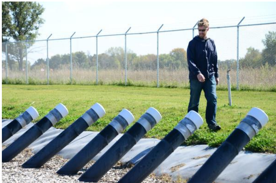
Ventilation Tubes at East Bethel WWTP. Source: Metropolitan Council Digital Image Library
