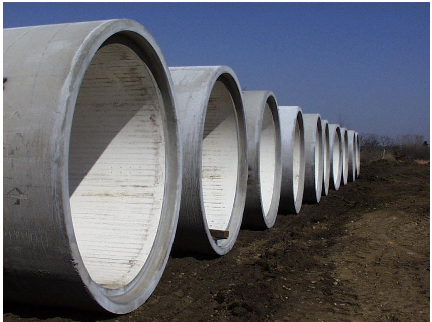
A row of interceptor pipes in south Washington County. Source: Metropolitan Council Digital Image Library
