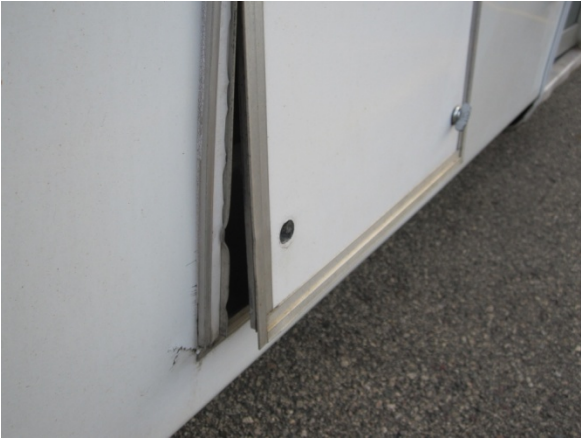
Fig 5.1 Missing panel /exposed wires
