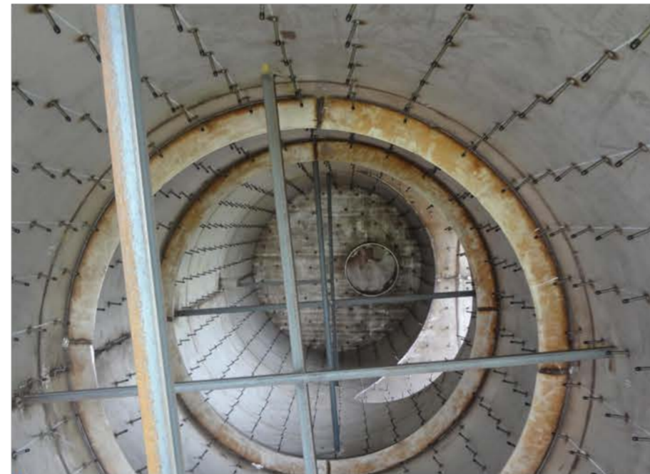
SS Crossover Ducts
