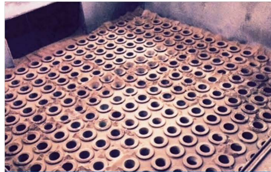
SS Baghouse Covers
