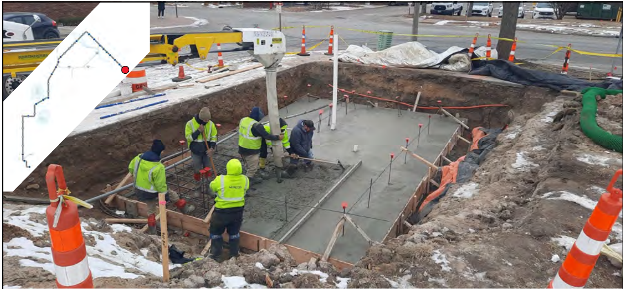
Westgate Station driver facility, January 2025
