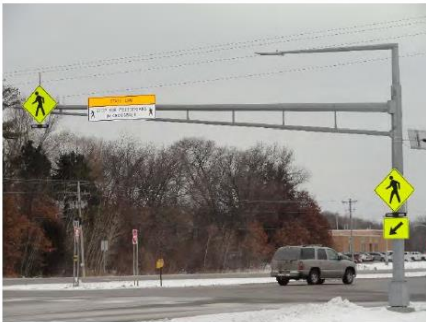
Figure 6: Rectangular Rapid Flash Beacons at Highway Crossing
