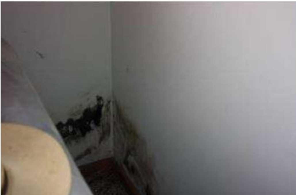
Figure 4: Mold in lower bedroom
