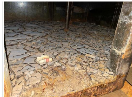
Photograph #10 75 Bidwell Building/Farwell Yards Redevelopment B1900287.06 Date: December 22, 2020 Direction: South Subject: Residual hardened resin, inactive AST, basement
