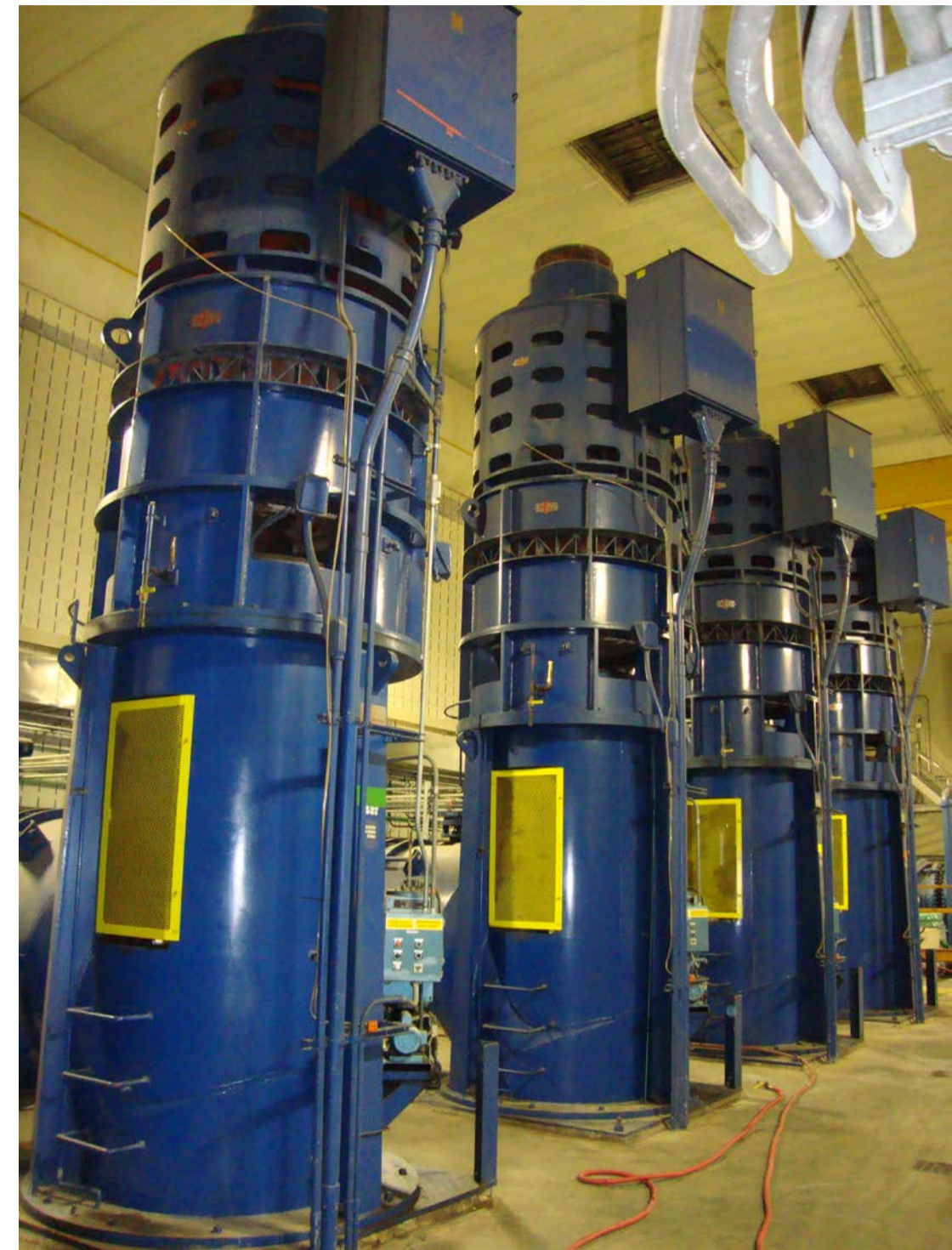
Effluent Pumping Station
