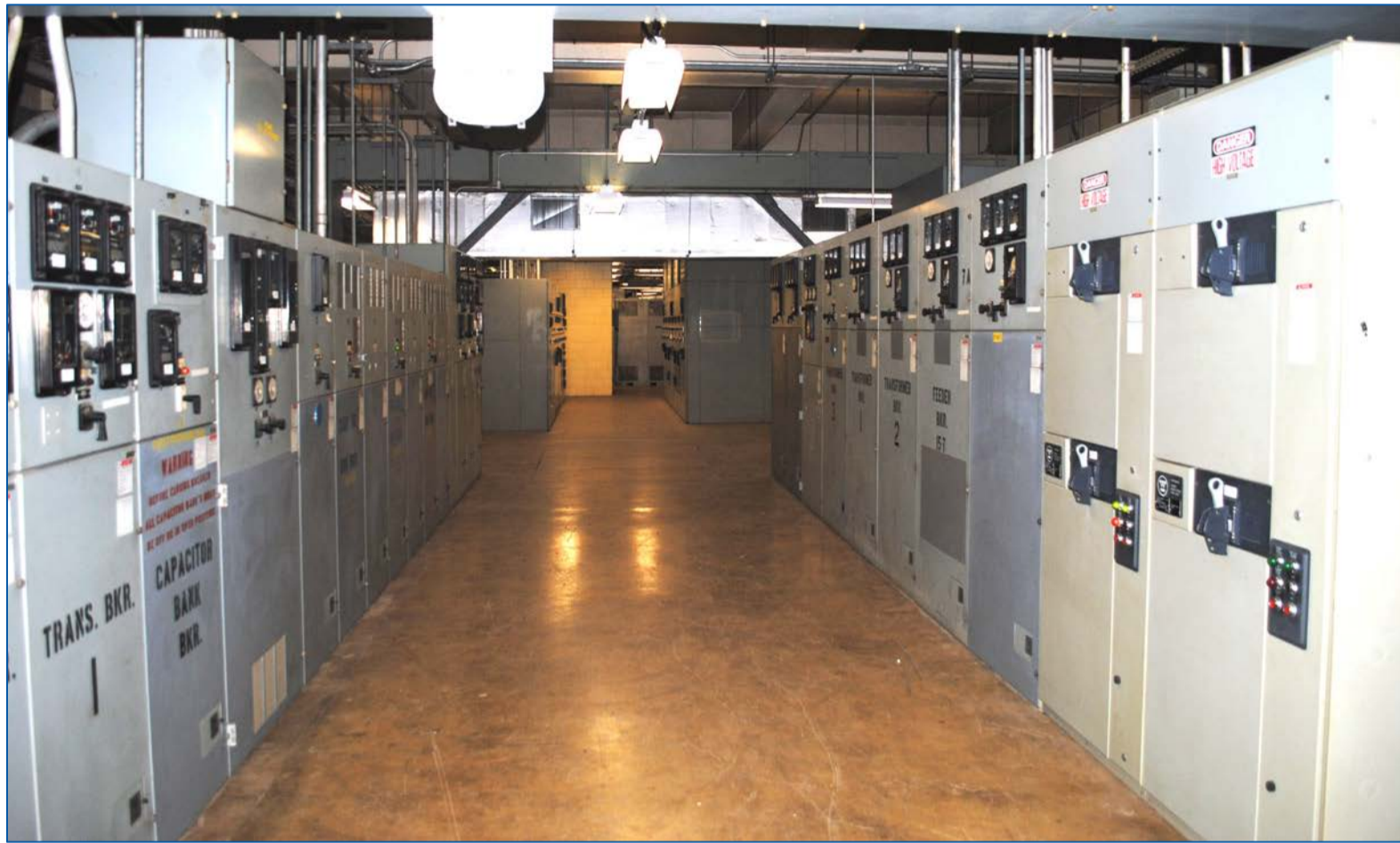
Switchgear Lineup in the Compressor Building
