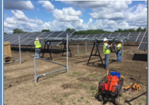
Solar panel installation at the Blue Lake Plant in Shakopee. The panels became operational in March 2016.
