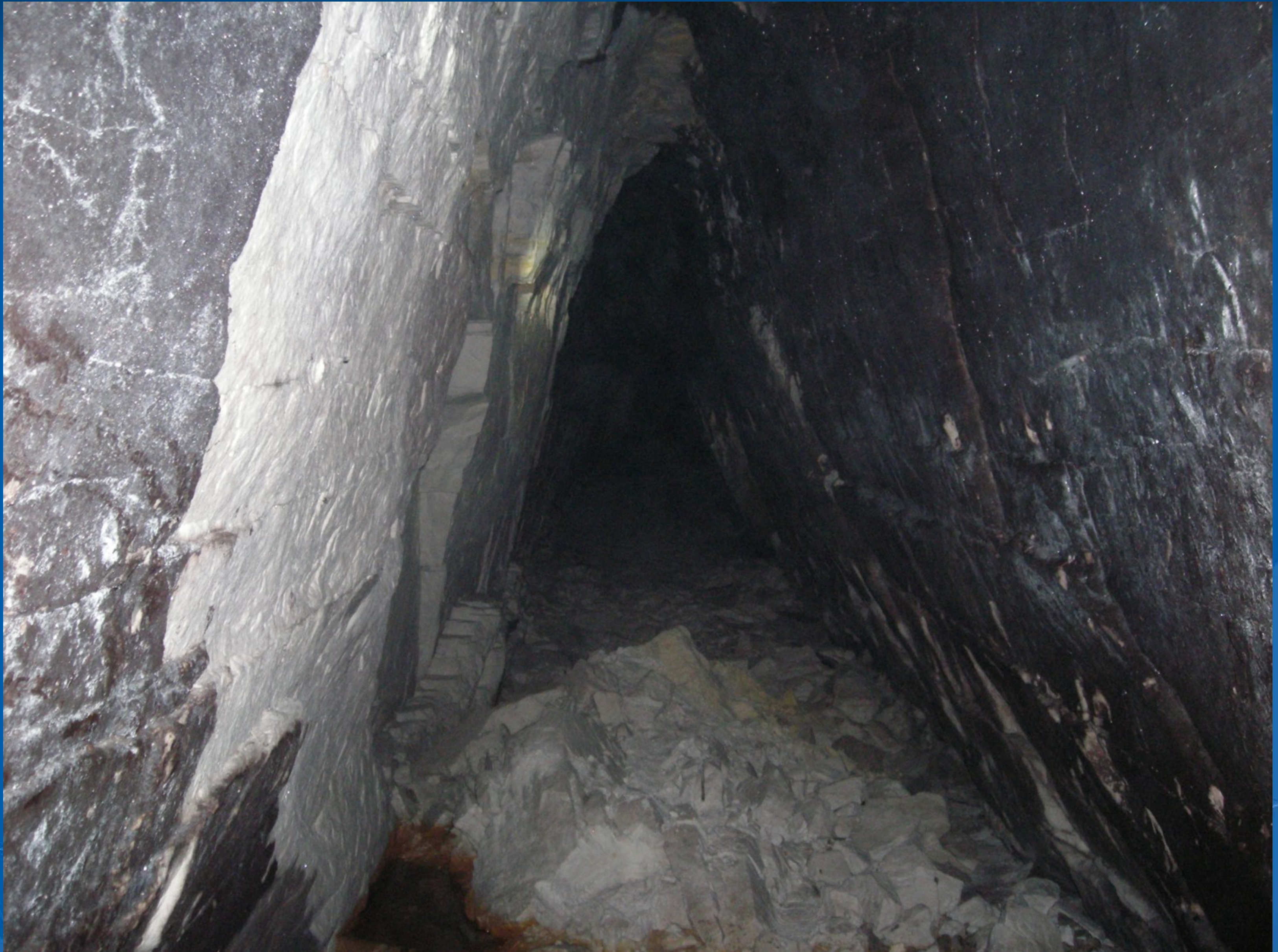
Void above Interceptor 1-MN-320 80 feet beneath 4th St. in downtown Minneapolis
