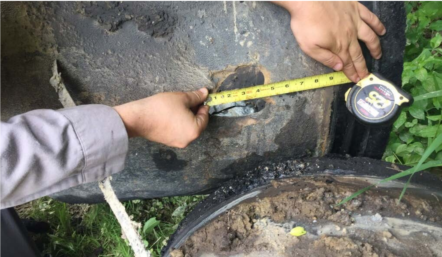
Photo showing size of hole in forcemain ~ 4.5” in diameter
