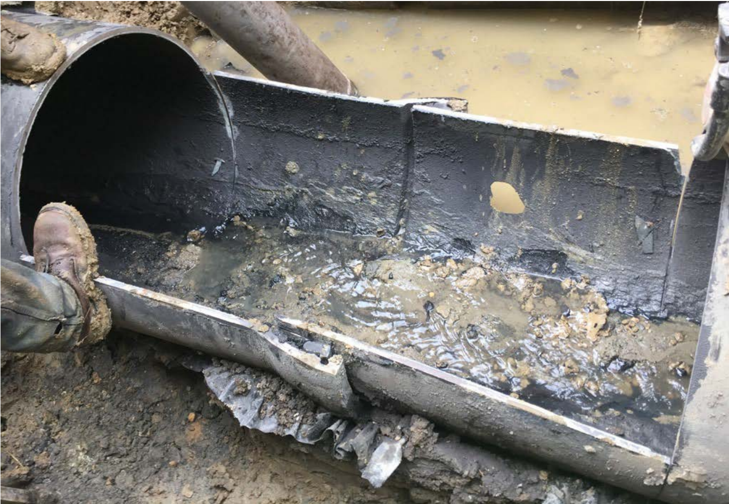
Cut-away of damaged pipe section prior to repair showing hole in pipe that was source of sewage release
