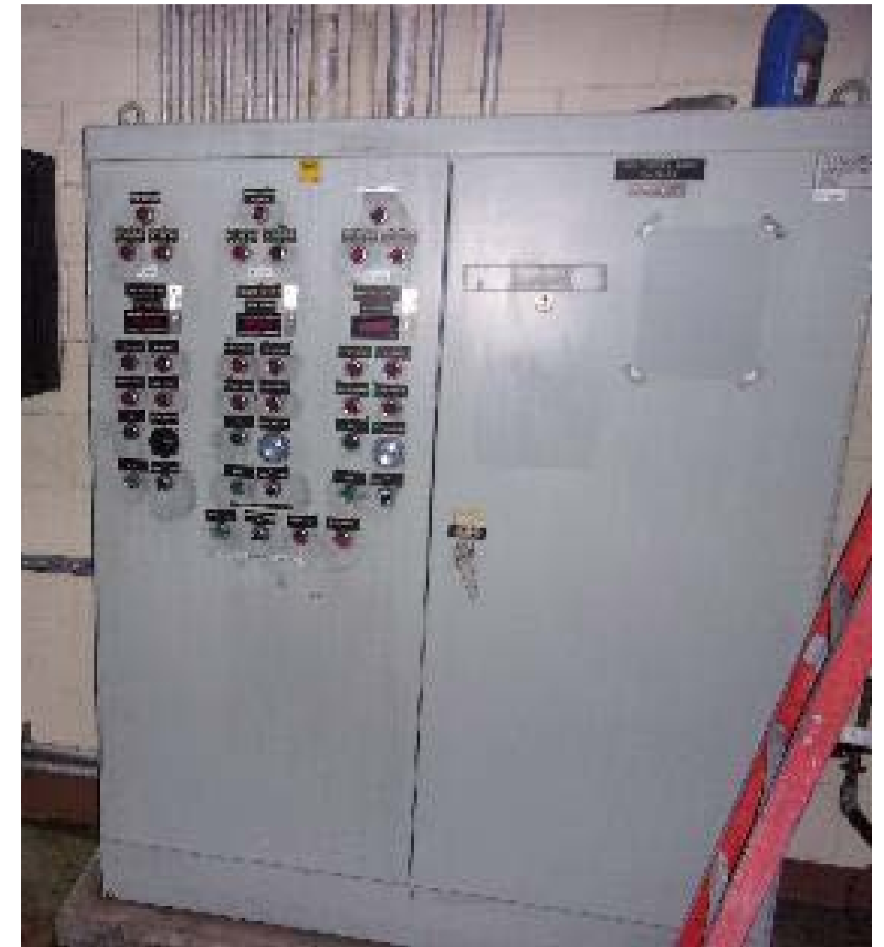
Obsolete Control Cabinet
