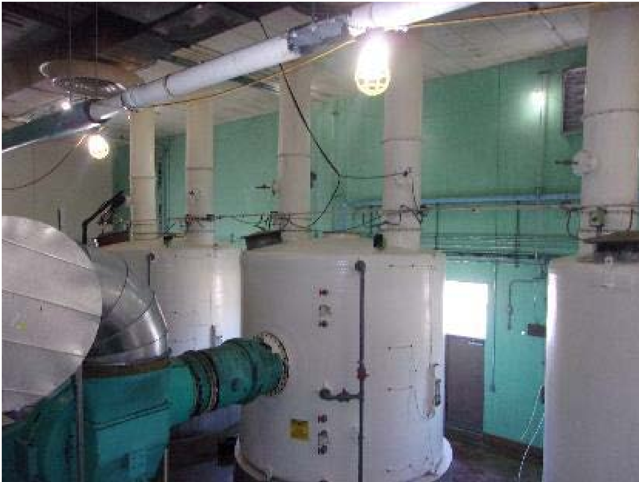
Odor Control Vessels
