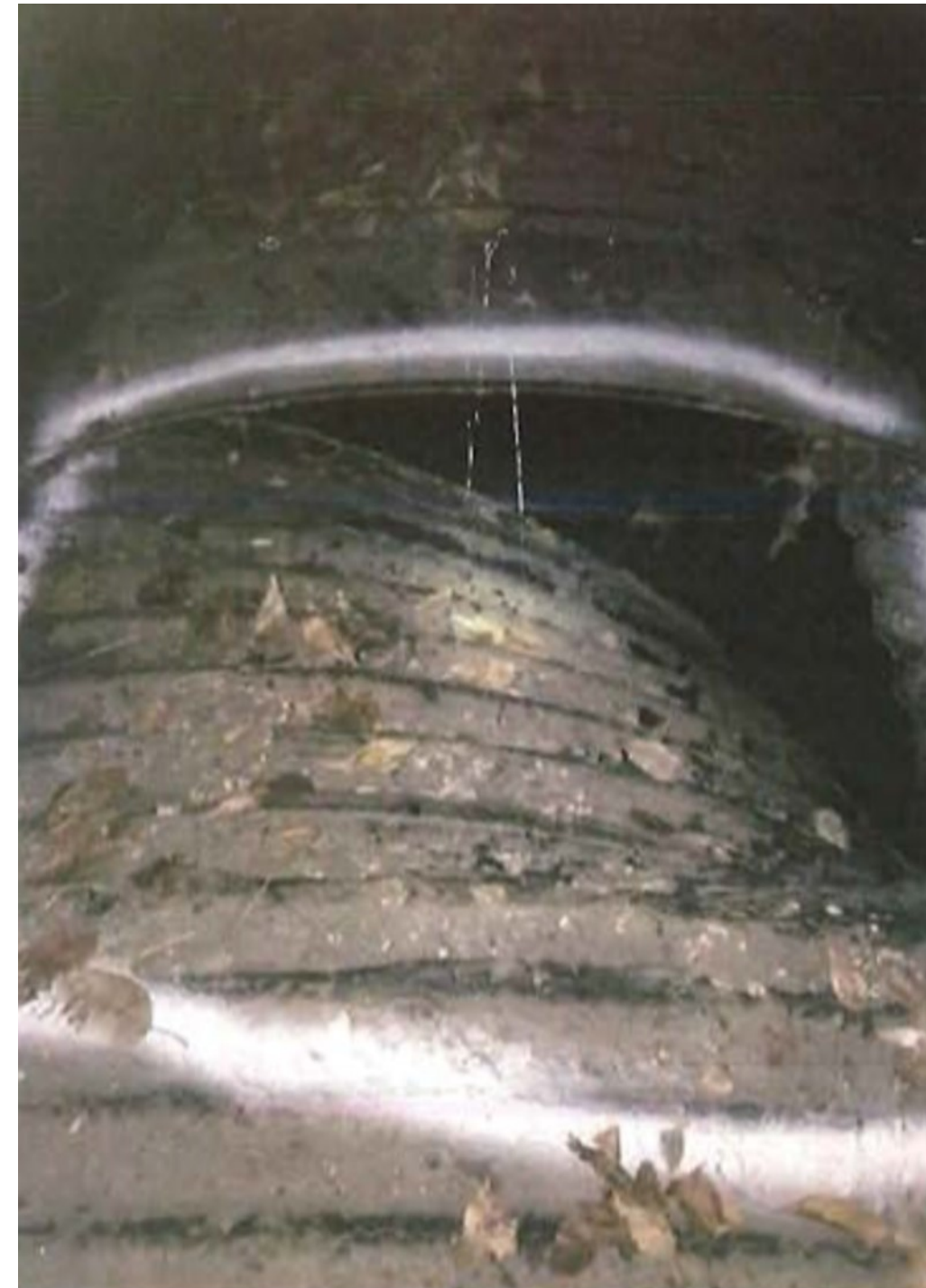
Pipe in pipe damage
