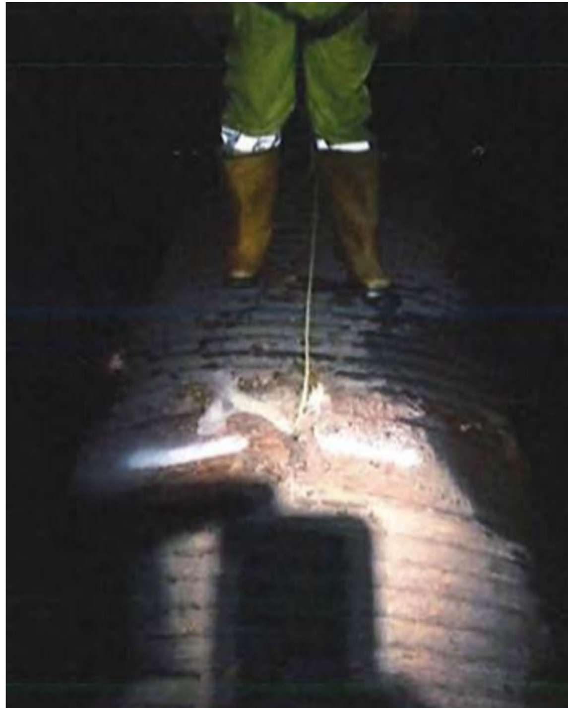
Pipe in pipe
