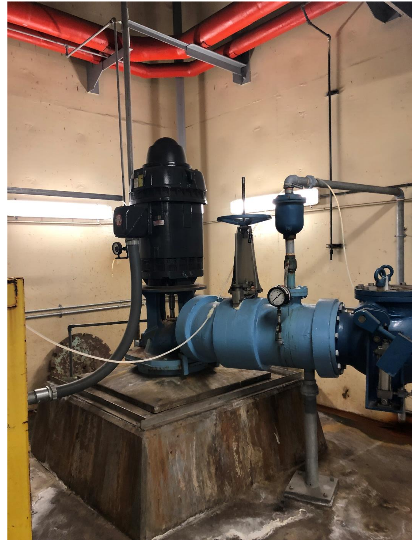
Metro Plant Service Water Pump
