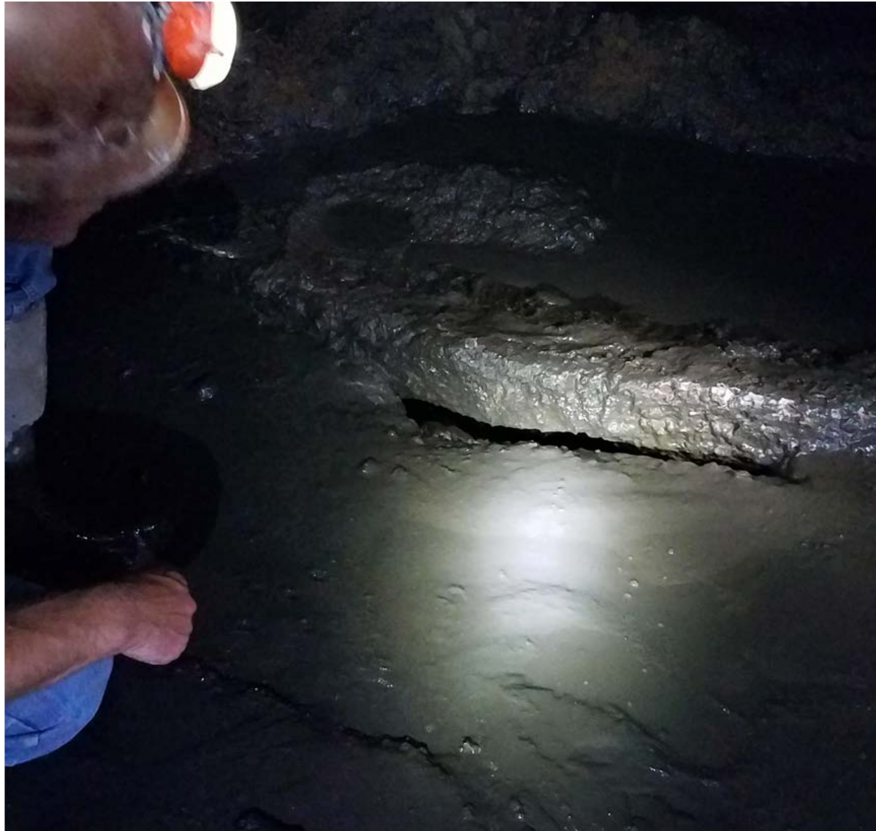
Crack and Heave
