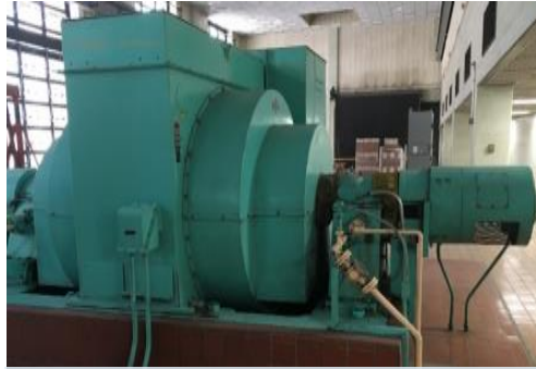
Compressor Motor Rehab Phase 2
