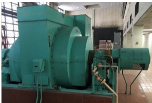
Compressor Motor Rehab Phase 2
