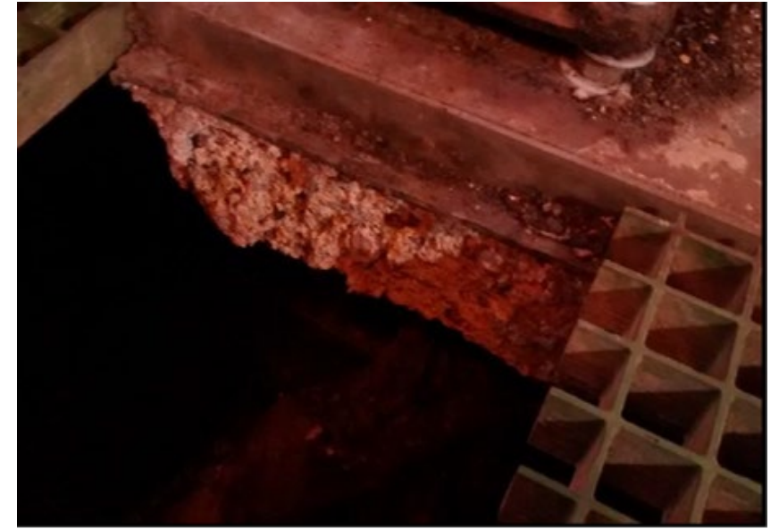
L66's Corroded Concrete Wetwell (2018)
