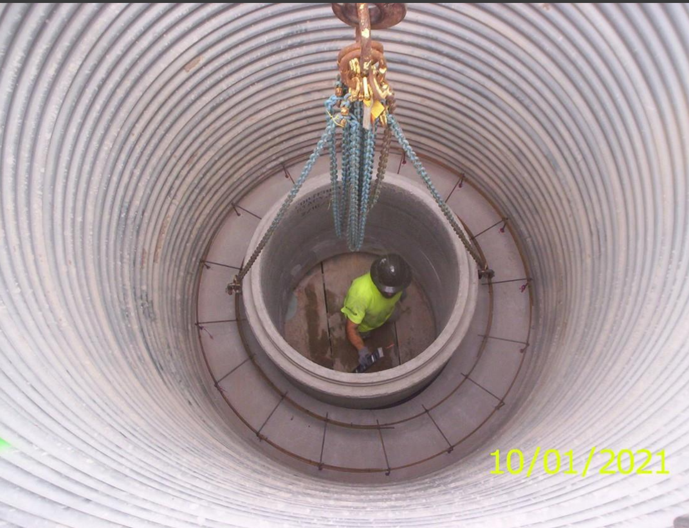
Corrugated pipe used to form inside of concrete outer structure with new internal access riser formed over pipe
