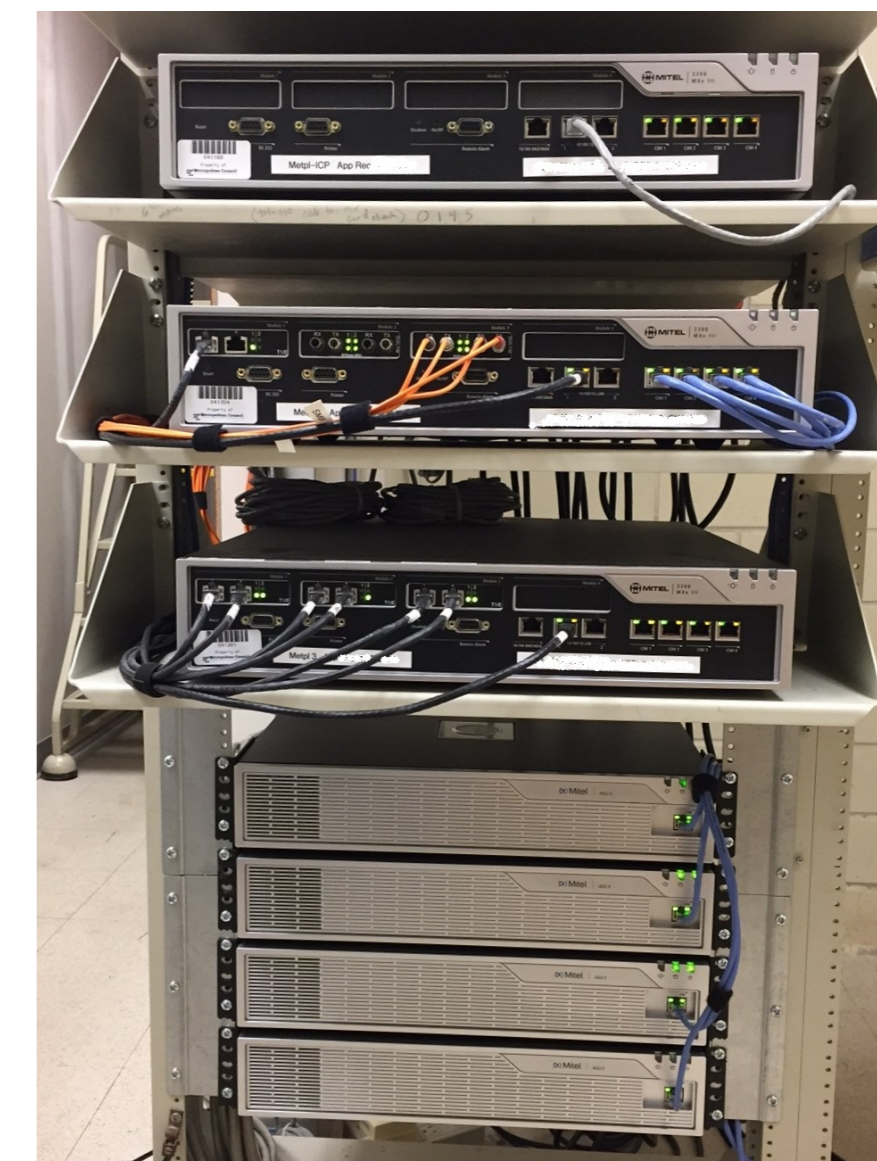
Metro Plant Controllers
