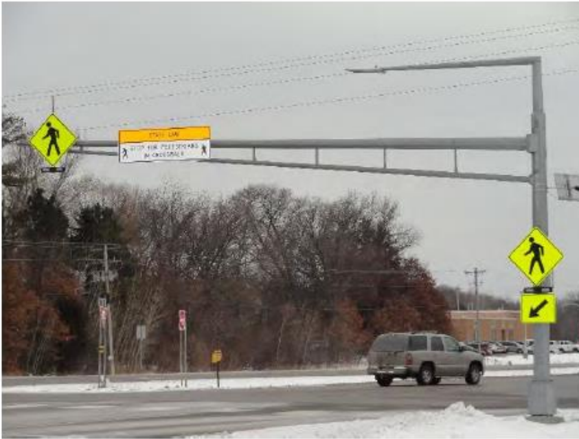
Figure 6: Rectangular Rapid Flash Beacons at Highway Crossing
