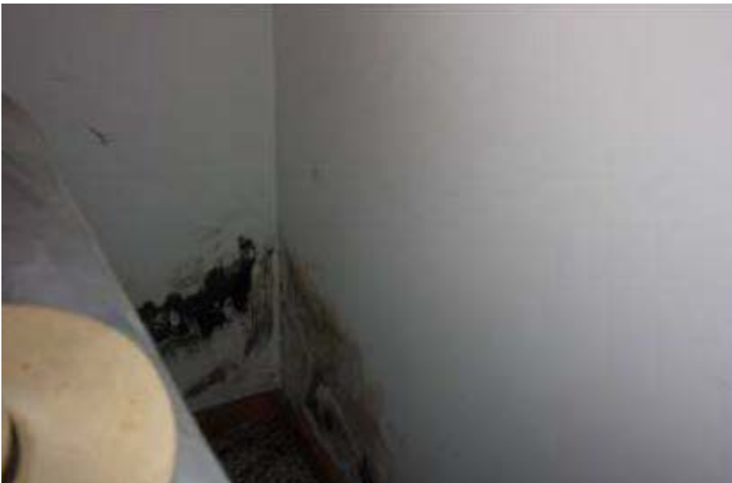
Figure 4: Mold in lower bedroom
