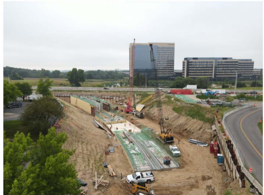
The construction of the LRT tunnel under Highway 62 is a multi-year process. With traffic shifted onto one side of the Highway crews have built the base of the tunnel and are working to progress walls and roofing.
