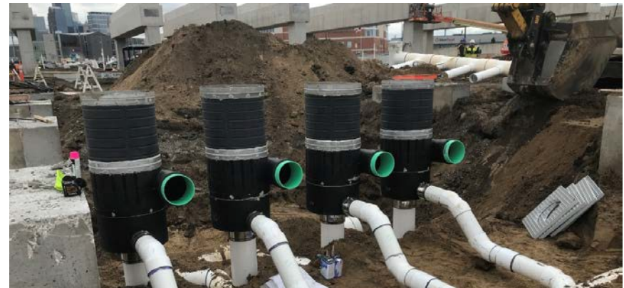
Rainwater filtration system for bus wash (Fall 2020)
