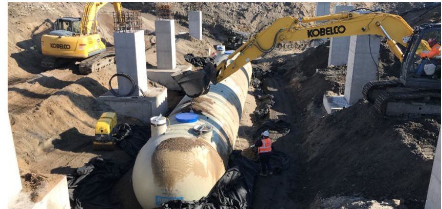
40,000 gallon rainwater storage tank (Fall 2020)
