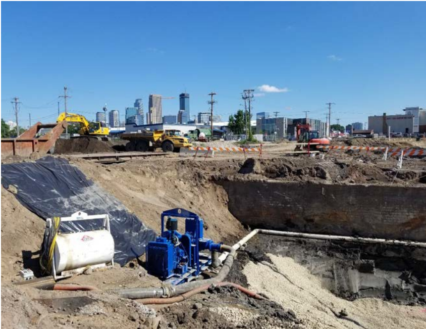
Dewatering pumps and piping – DBE
