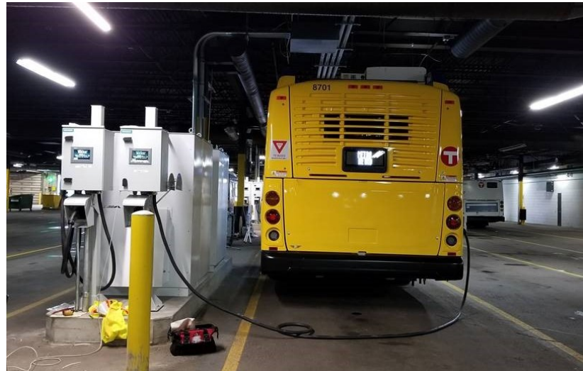
Figure 15: Siemens RAVE 150 plug-in chargers at the Heywood Garage
