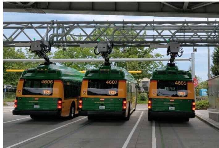
Figure 21: King County Metro overhead gantry charging system
