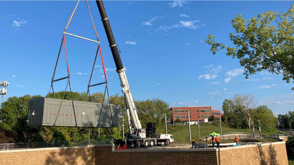
TPSS SW306 Installation in Minnetonka
