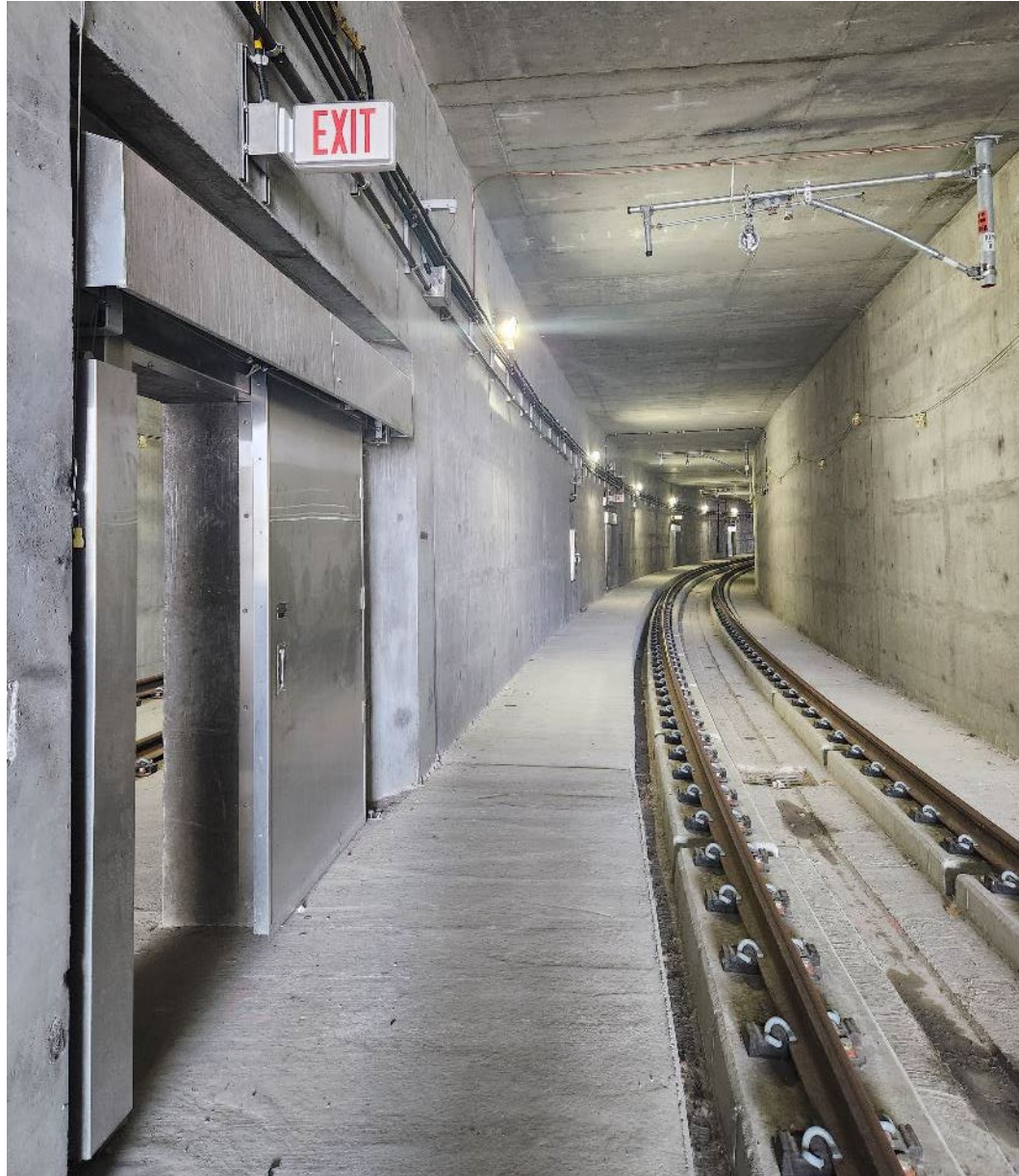
Lighting in TH62 LRT tunnel
