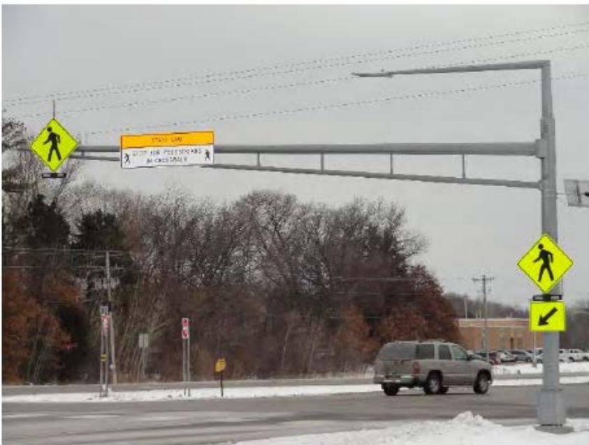
Figure 6: Rectangular Rapid Flash Beacons at Highway Crossing
