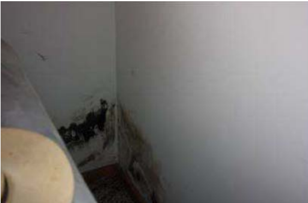
Figure 4: Mold in lower bedroom
