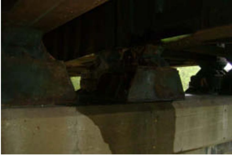
Pier 6: Drainage on to Pier from Deck
