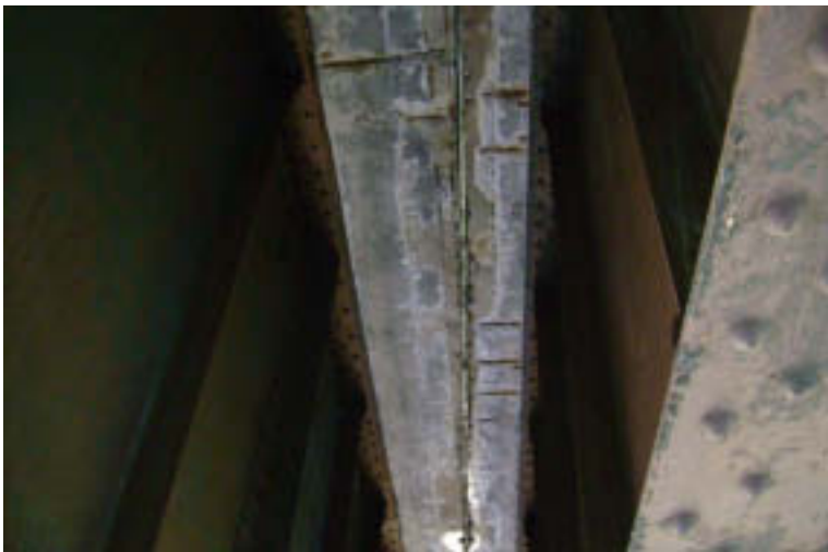
Span 5: Expose Reinforcement
