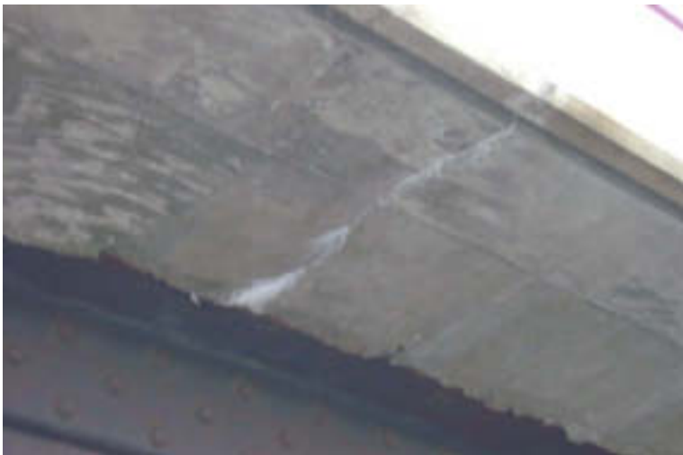
Span 4: Deck Crack and Bleaching
