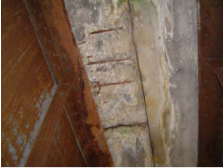
Span 2: Exposed Reinforcement
