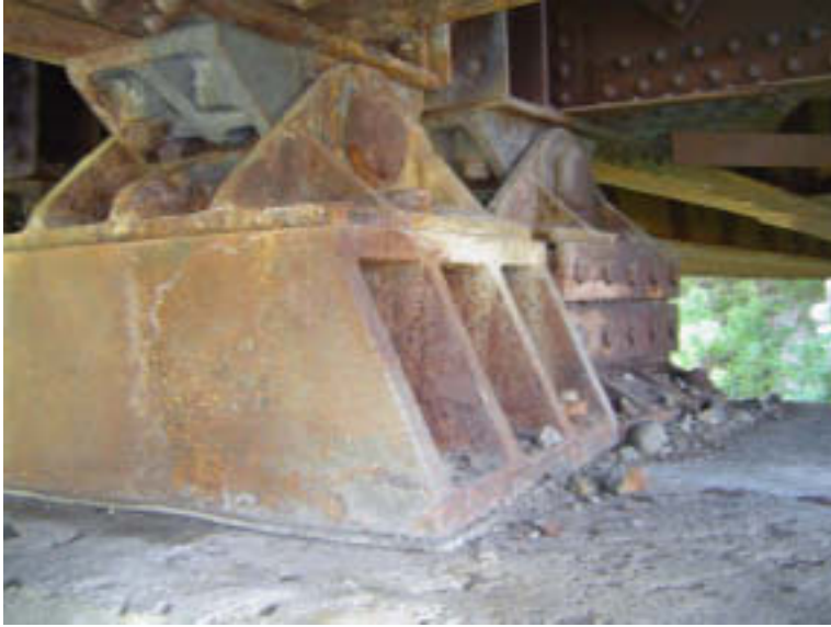
Pier 7: Bearing Calcium Carbonate
