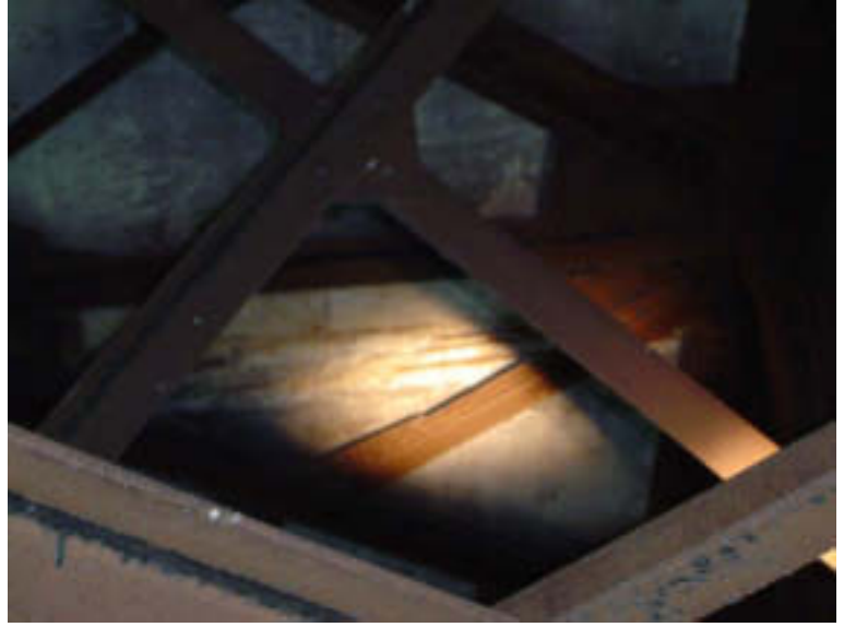
Span 7: Expose Reinforcement
