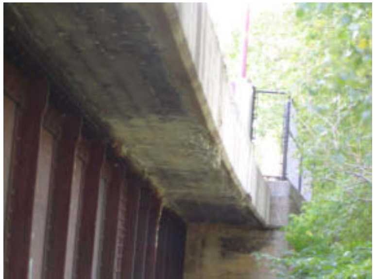
Span 7: Calcium Carbonate Built Up
