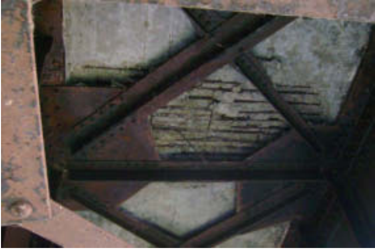
Span 1: Exposed Reinforcement
