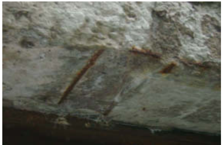
Span 6: Deck Expose Reinforcement
