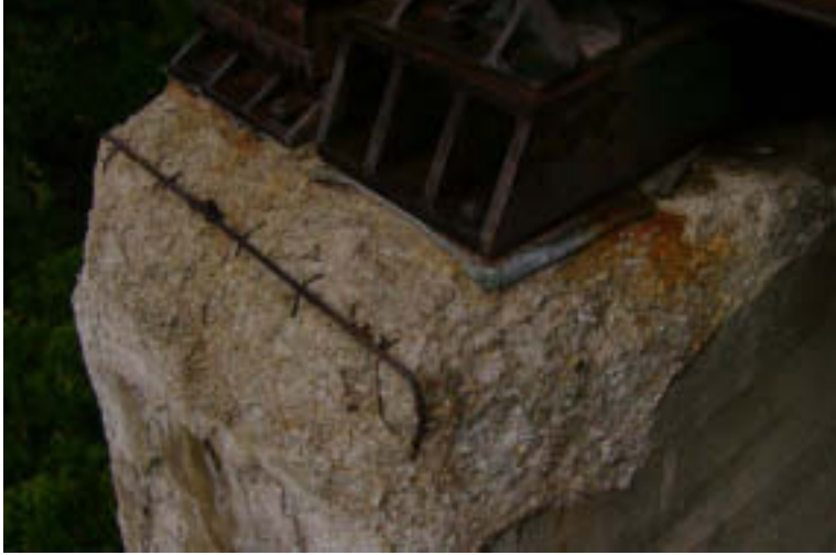
Pier 7: Pier Cap Deterioration
