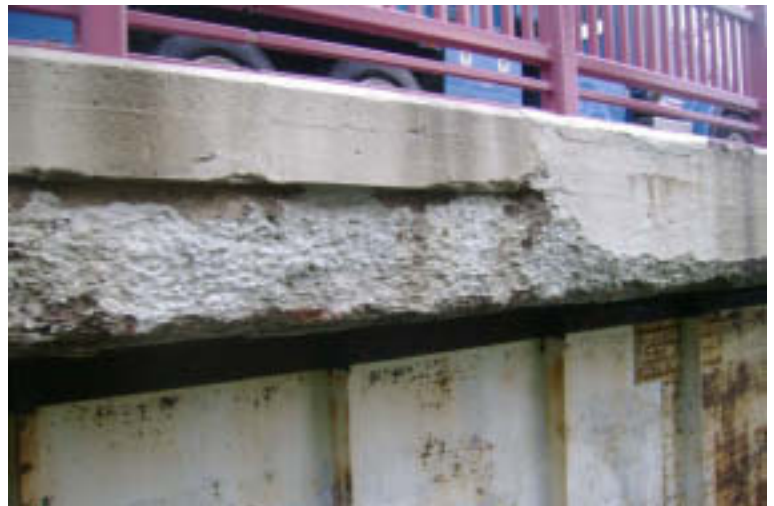
Span 7: Deck Spawling
