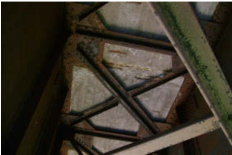
Span 6: Deck Expose Reinforcement
