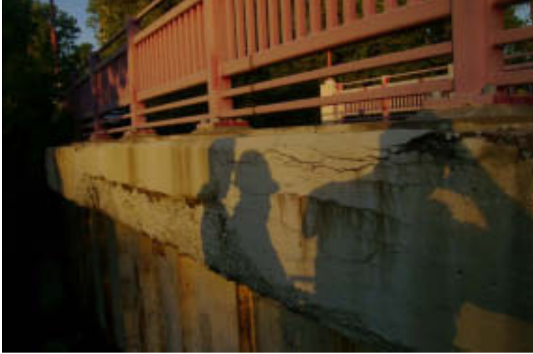
Span 7: Deck Weathering
