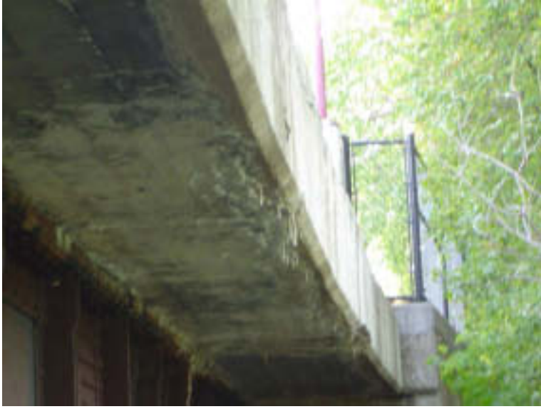
Span 7: Calcium Carbonate Built Up
