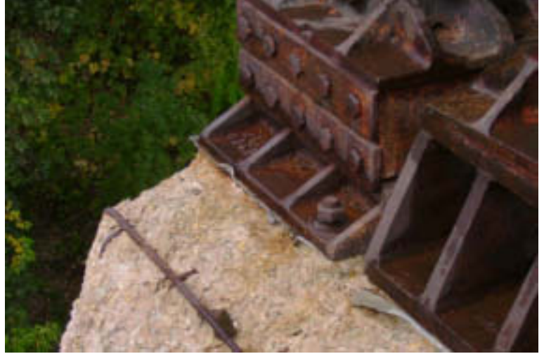
Pier 7: Pier Cap Deterioration
