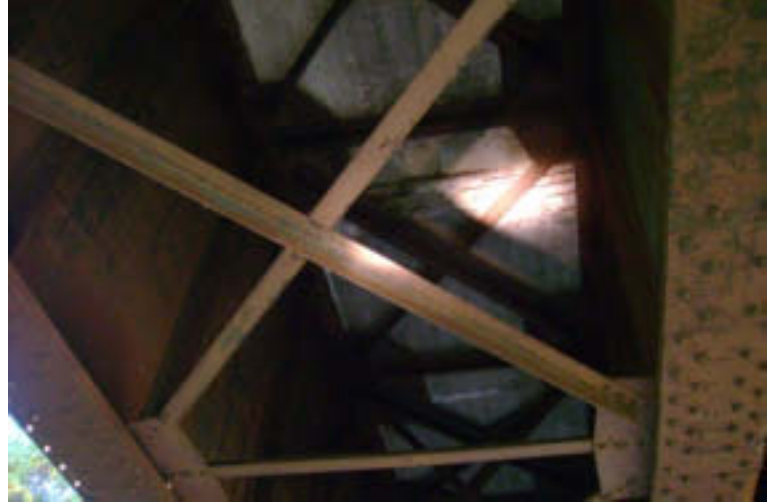
Span 7: Deck Exposed Reinforcement
