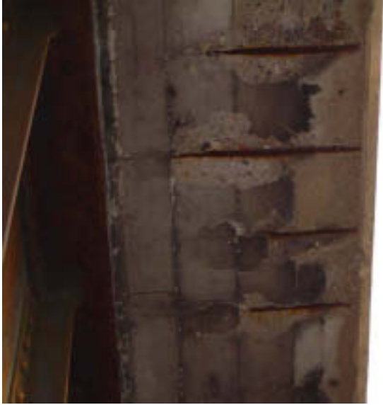
Span 1: Soffit Exposed Reinforcement
