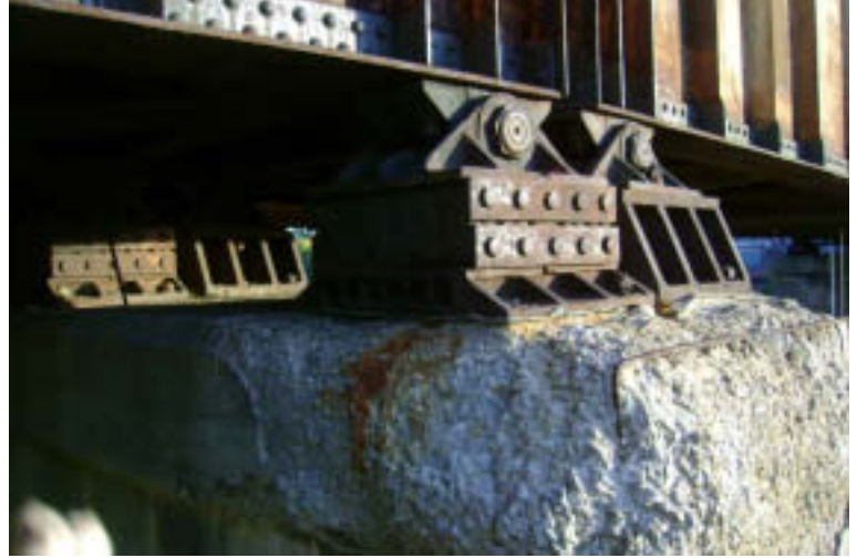
Pier 7: Pier Cap Deterioration
