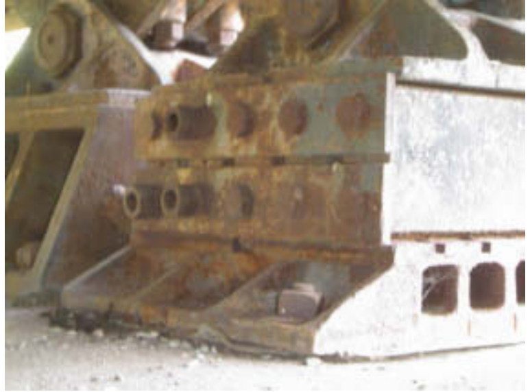
Pier 6: Bearing and Calcium Carbonate
