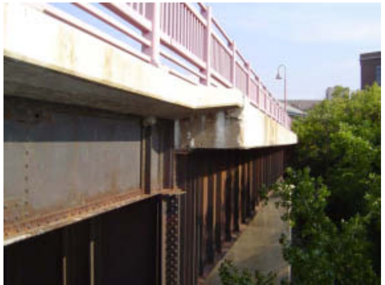
Span 2: Staining from Drainage
