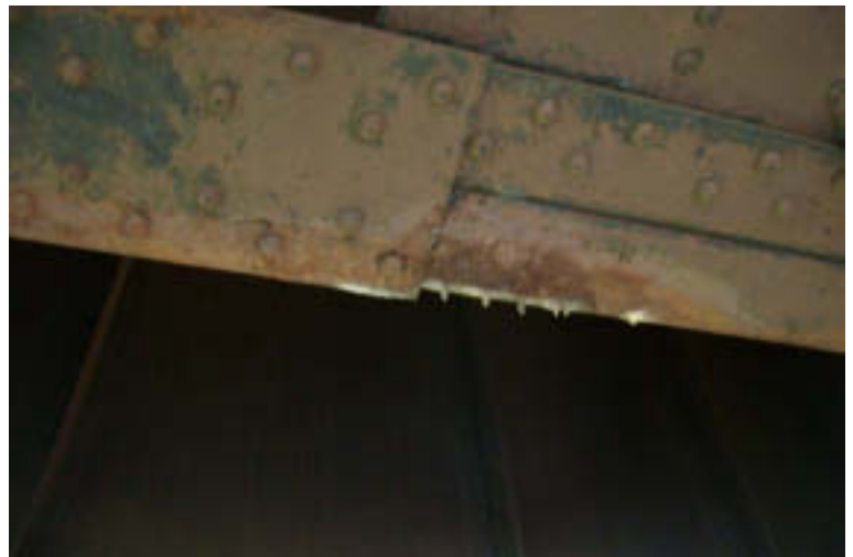
Span 5: Calcium Carbonate Dripping
