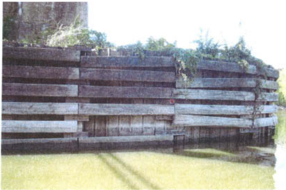
Photograph 2. View of Damaged Fender System at Upstream Half of Pier 4, Looking West.
