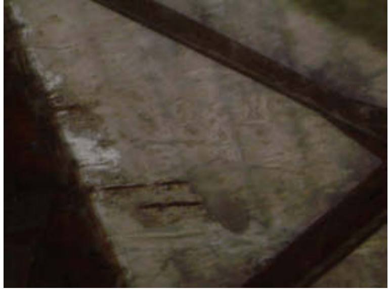
Span 2: Exposed Reinforcement
