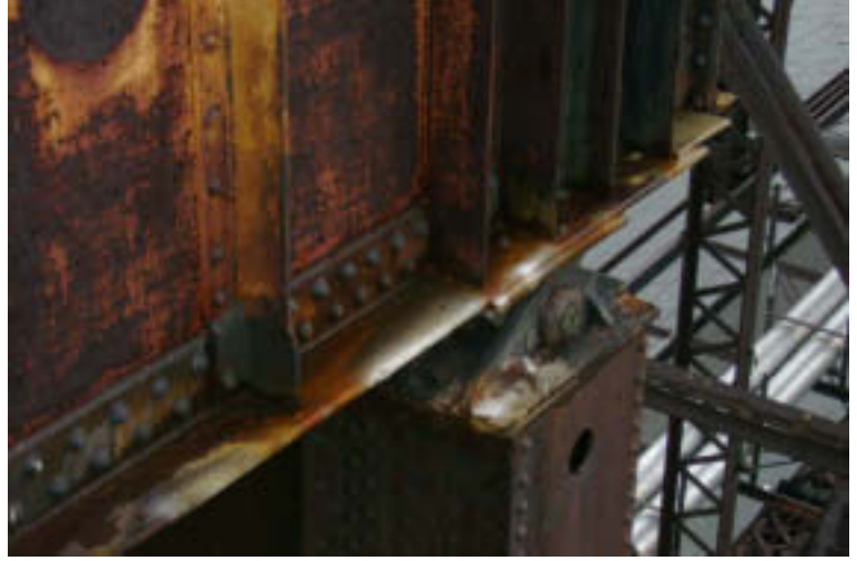
Pier 5: Steel Cap Calcium Carbonate Built Up
