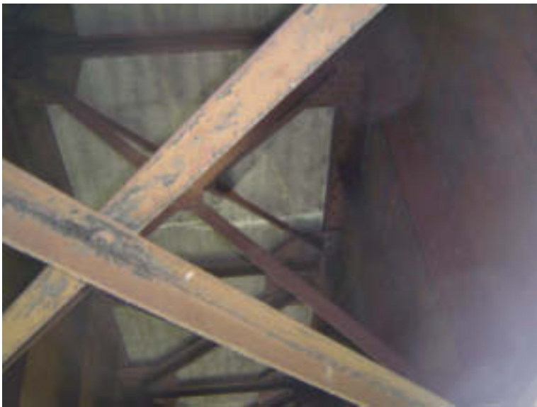
Span 6: Deck Crack
