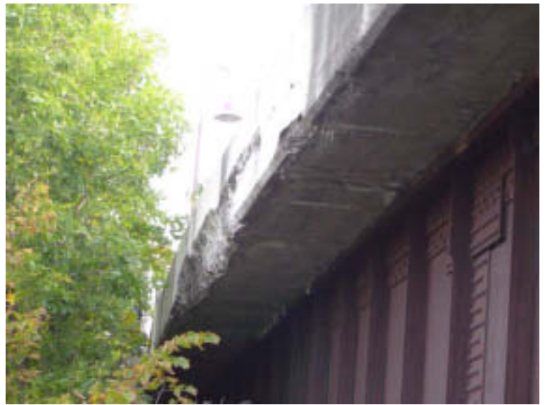
Span 1: Soffit Exposed Reinforcement
