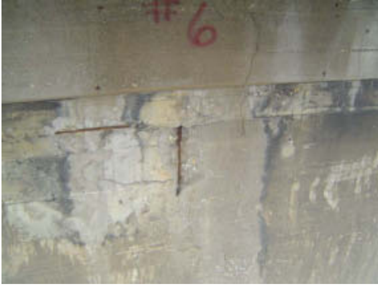
Pier 6: Exposed Reinforcement Below Cap
