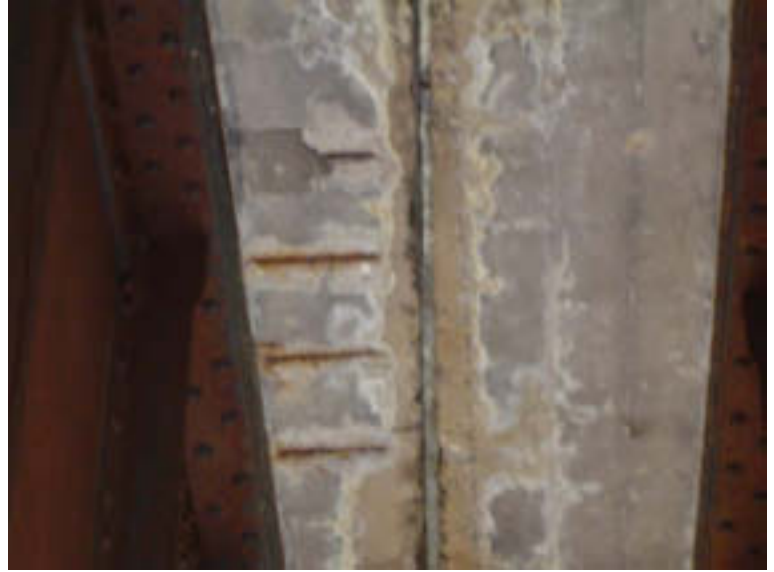
Span 6: Deck Expose Reinforcement
