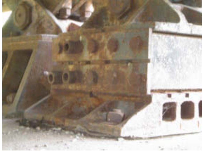
Pier 6: Bearing and Calcium Carbonate
