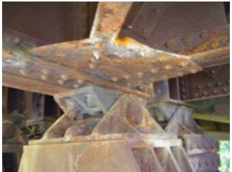
Pier 7: Bearing Calcium Carbonate
