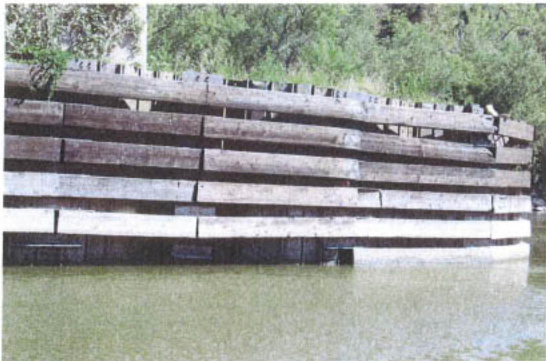
Photograph 4. View of the Damaged Fender System at Downstream Half of Pier 4, Looking East.
