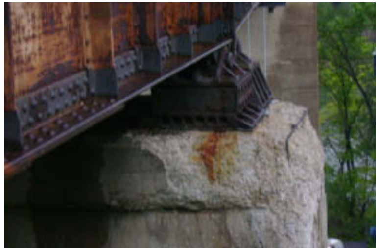
Pier 7: Pier Cap Deterioration
