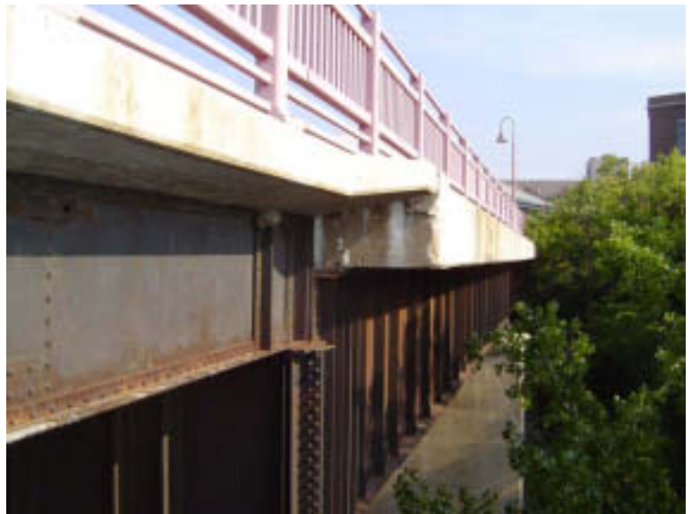
Span 2: Staining from Drainage
