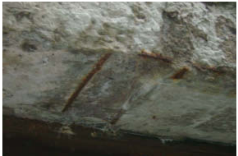
Span 6: Deck Expose Reinforcement
