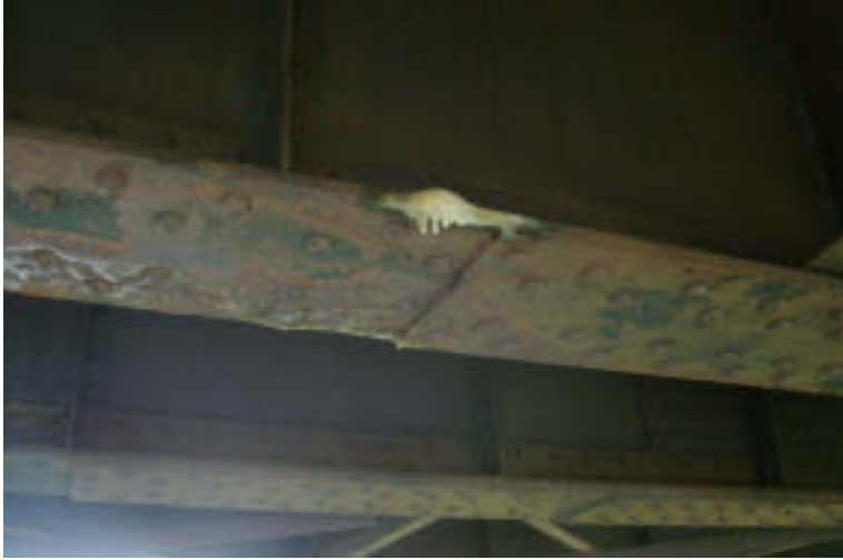
Span 5: Calcium Carbonate Build Up
