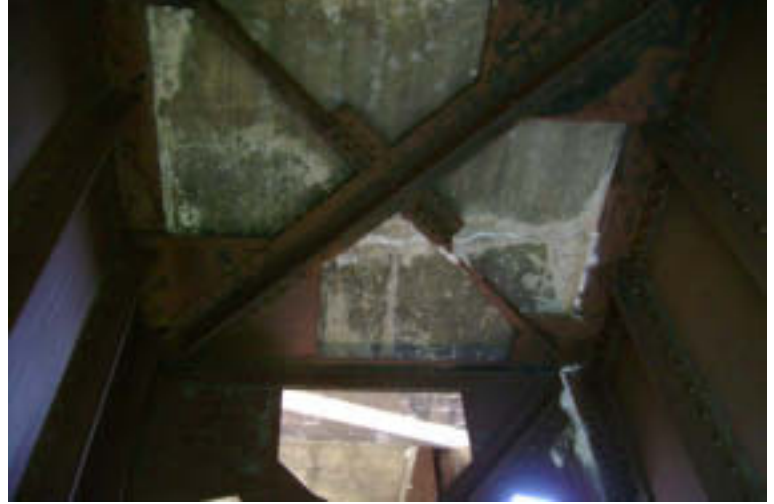
Span 5: Calcium Carbonate Dripping from Deck to Girders
