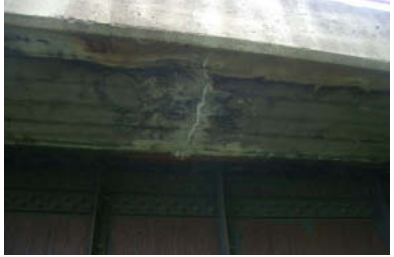
Span 1: Soffit Crack
