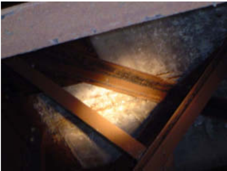
Span 7: Expose Reinforcement
