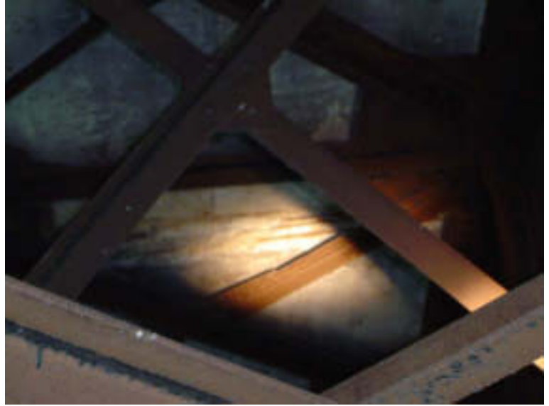
Span 7: Expose Reinforcement
