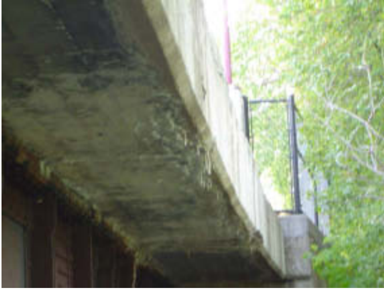
Span 7: Calcium Carbonate Built Up
