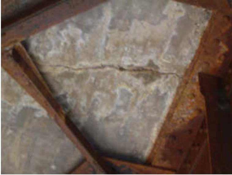
Span 6: Drainage Cracks
