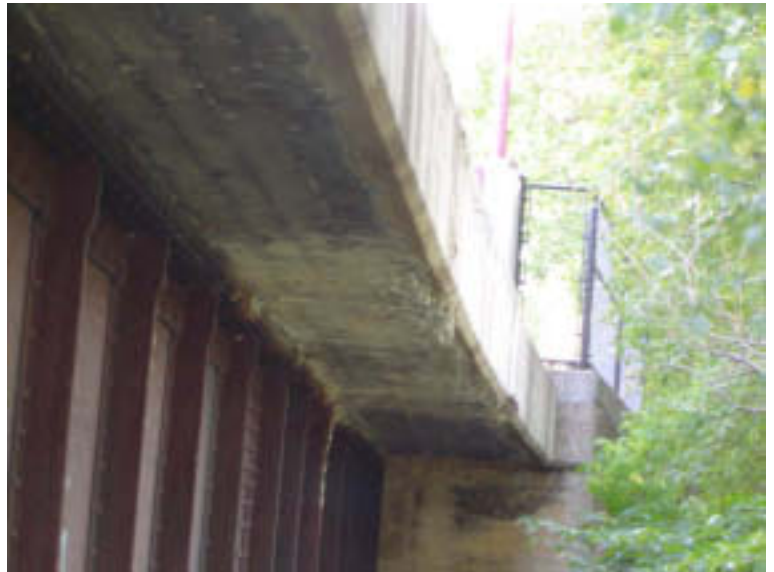
Span 7: Calcium Carbonate Built Up
