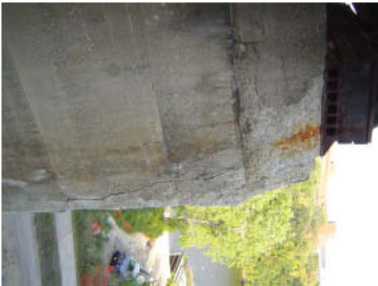
Pier 7: Pier Cap Deterioration
