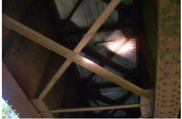
Span 7: Deck Exposed Reinforcement
