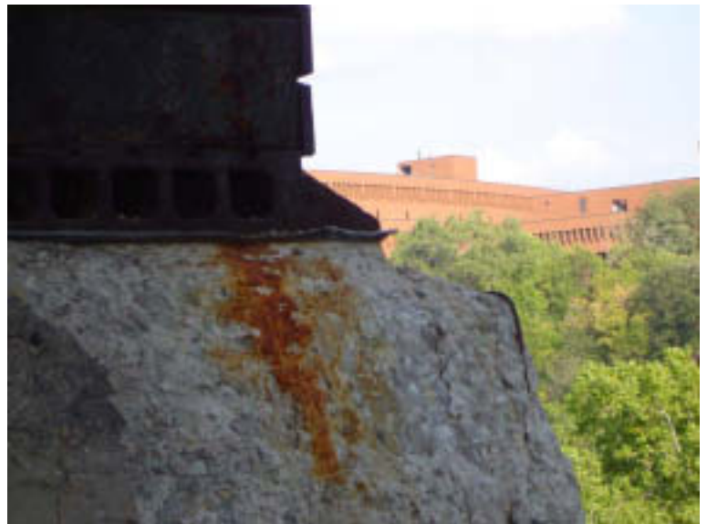
Pier 7: Pier Cap Deterioration
