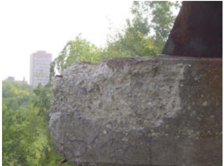
Pier 6: Pier Cap Deterioration
