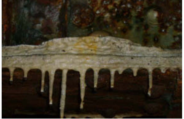
Span 7: Calcium Carbonate Built Up
