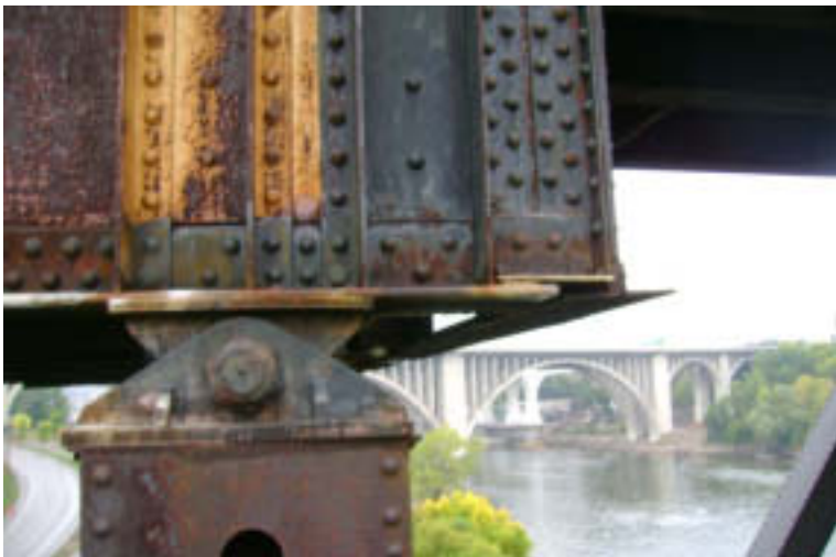
Pier 5: Steel Cap Calcium Carbonate Built Up
