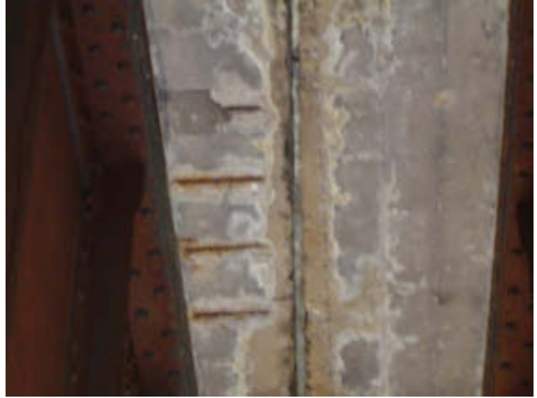
Span 6: Deck Expose Reinforcement
