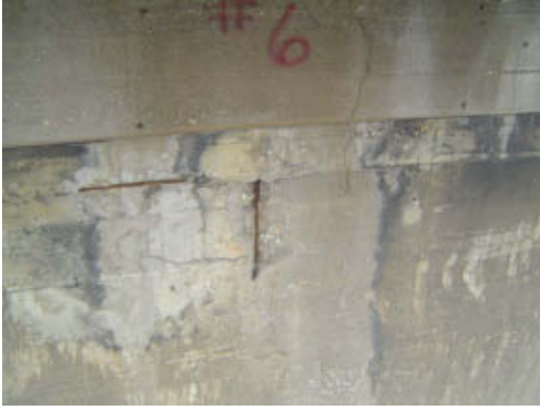
Pier 6: Exposed Reinforcement Below Cap
