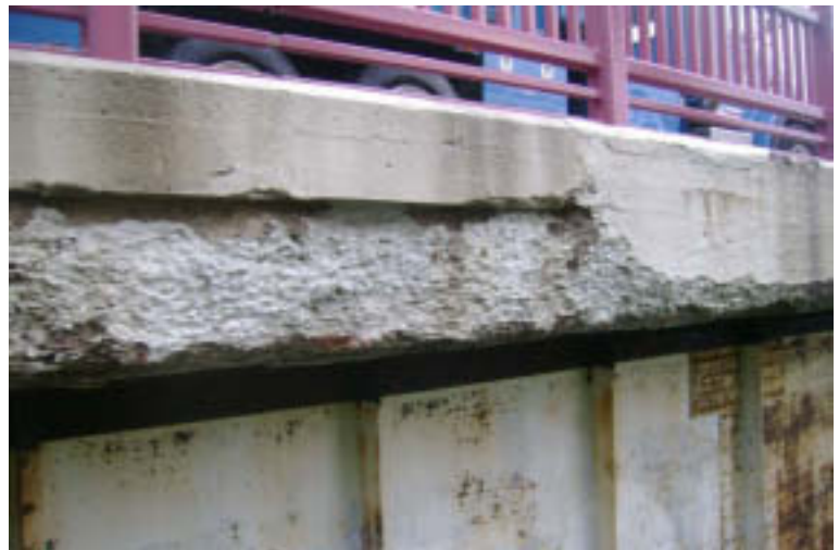
Span 7: Deck Spawling
