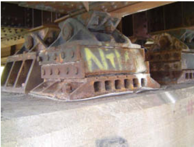
Pier 6: Bearing and Calcium Carbonate
