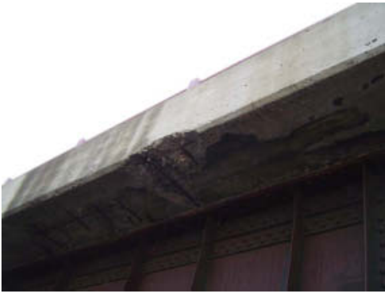
Span 1: Soffit Exposed Reinforcement
