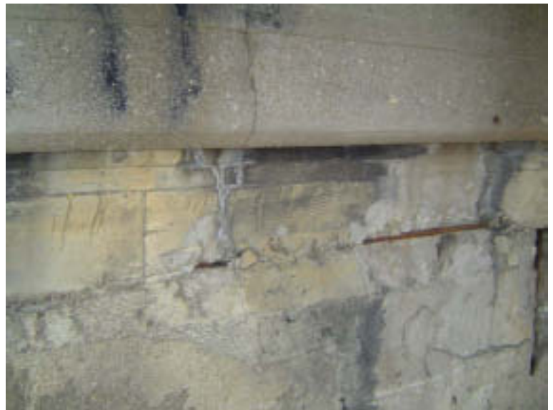
Pier 6: Exposed Reinforcement Below Cap
