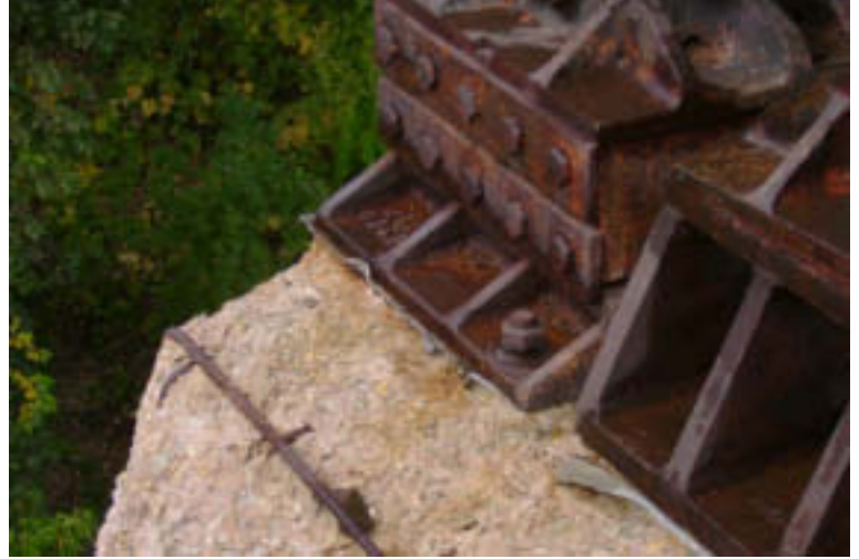
Pier 7: Pier Cap Deterioration
