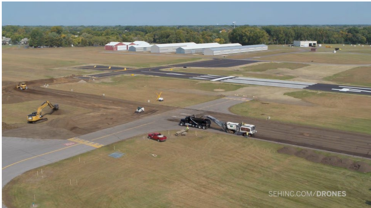
Photo of the Crystal Airport Runway 14R-32L and Taxiway E Modifications project construction.
