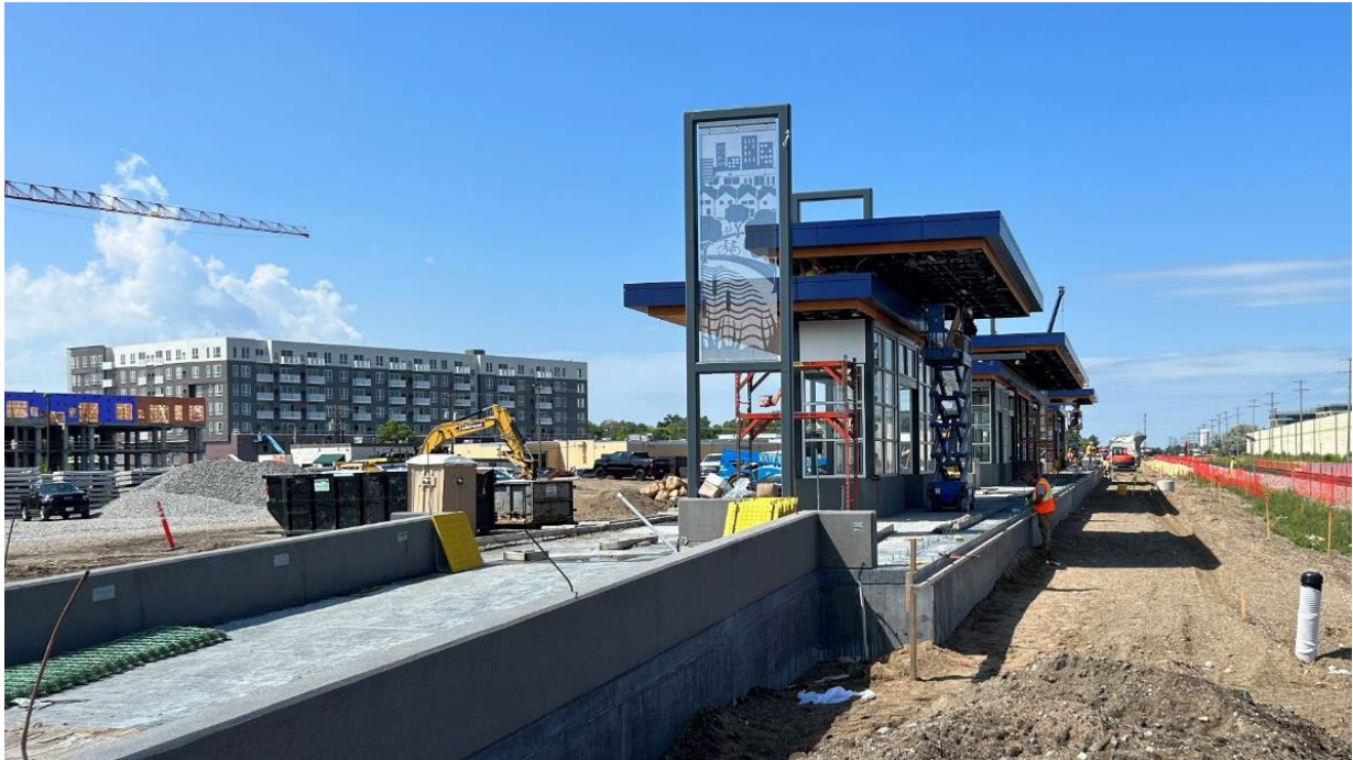
Blake Road Station
