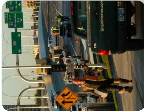
Figure 2-2: The increased cost of construction materials is just one challenge in maintaining transportation infrastructure.
