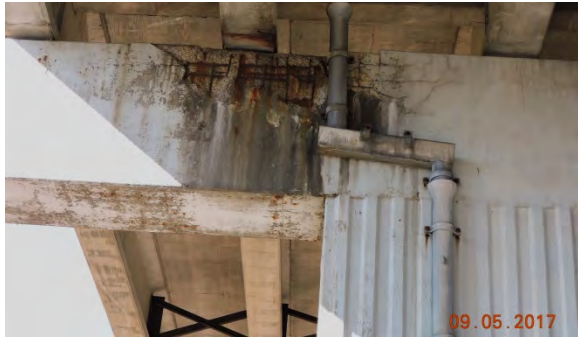
Photo 1. Cantilever pier cap cracking & deterioration. (no traffic loads can be supported by cantilevers)
