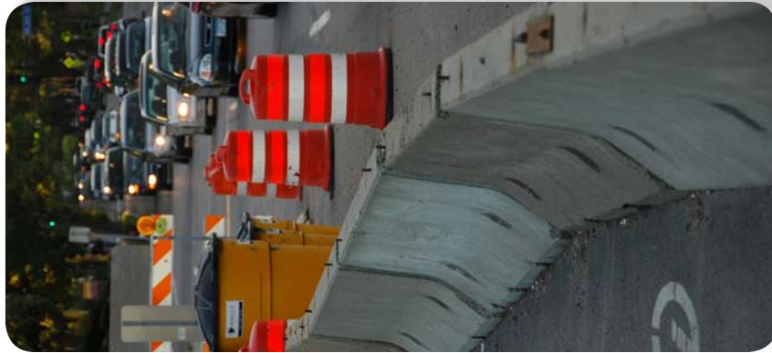
Figure 2-10: Road maintenance will continue to be a high priority in the region
