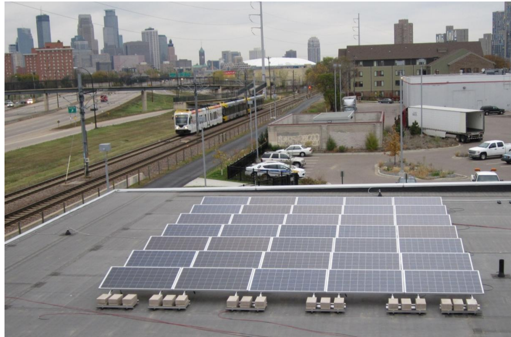
Solar array at Rail Support Facility
