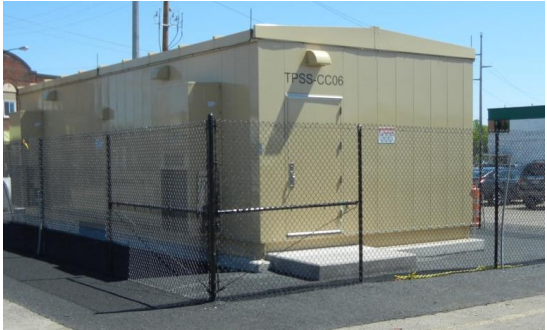
Traction power substation
