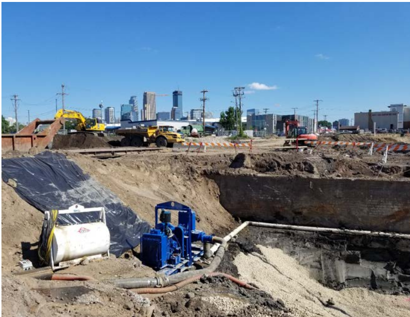
Dewatering pumps and piping – DBE
