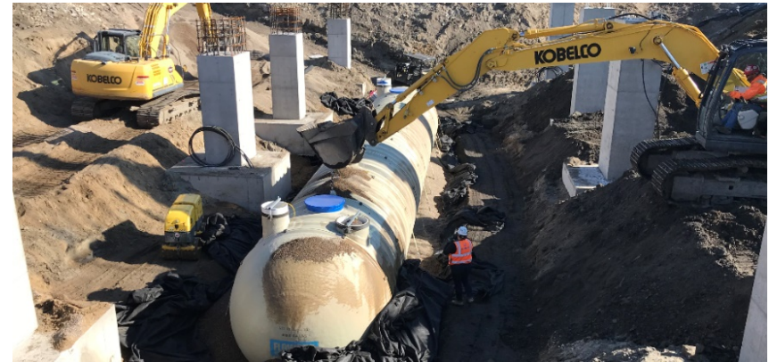
40,000 gallon rainwater storage tank (Fall 2020)
