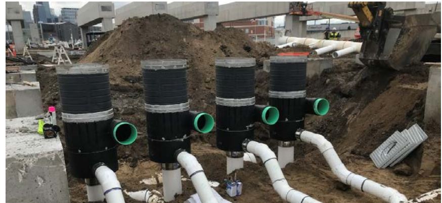
Rainwater filtration system for bus wash (Fall 2020)
