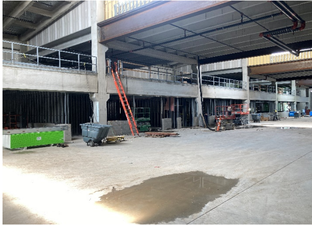
Mechanical Mezzanine Pre-Ductwork
