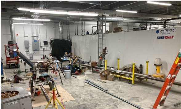
Diesel Fuel Tank
