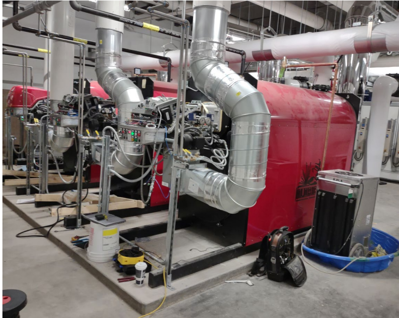
Boiler Heating System
