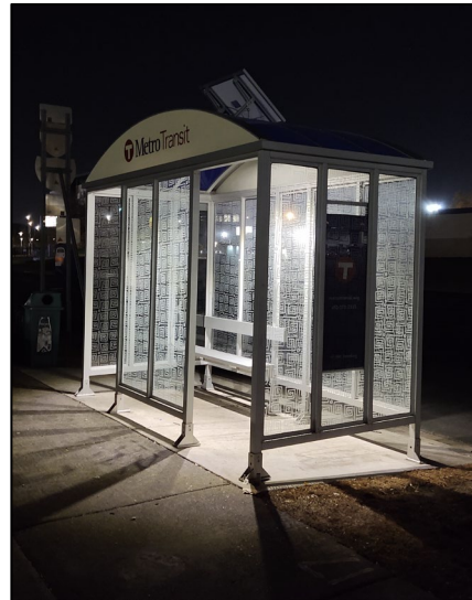
Rooftop mounted solar light (2022)
